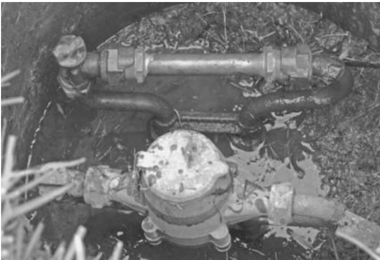
FIGURE 15.3 Bypassing a water meter is not complicated. This photo shows a “cheater” or “jumper” pipe (top) that was illegally used to replace the meter in the meter setter. In the lower part of this meter pit, is a typical 5/8-in residential meter. (Source: Morgantown Utility Board.)
