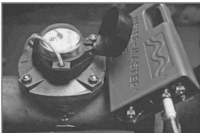
FIGURE C.3 Sensor attached to meter with Velcro strap. (Source: F. S. Brainard and Company.)
