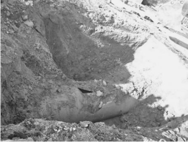
FIGURE 3.2 Transmission main break. (Source: WSO—Guido Wiesenreiter.)
