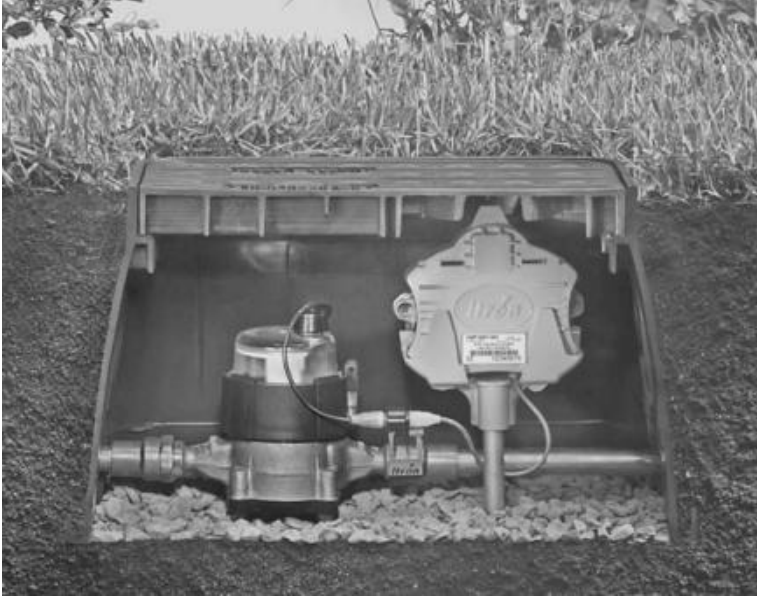
FIGURE 13.6 AMR endpoint device for residential meter in meter pit. (Source: Itron, Inc.)
