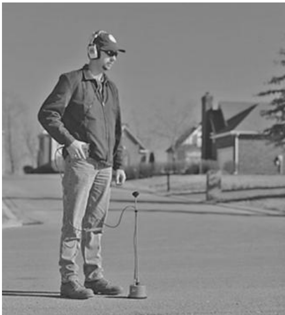
FIGURE B.36 Listening for leaks using an electronic geophone. (Source: Health Consultants, Inc.)
