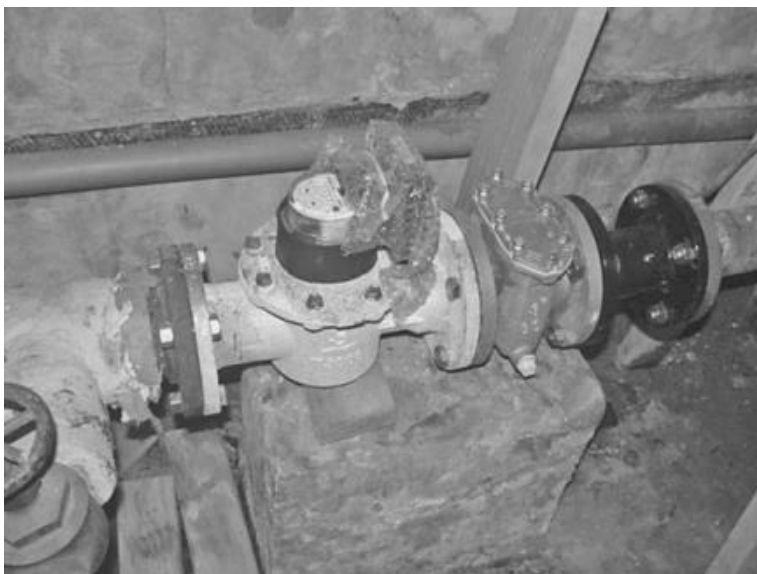
FIGURE 13.1 Indoor 3-in turbine meter servicing a 100-unit apartment building in Philadelphia. (Source: Philadelphia Water Department.)
