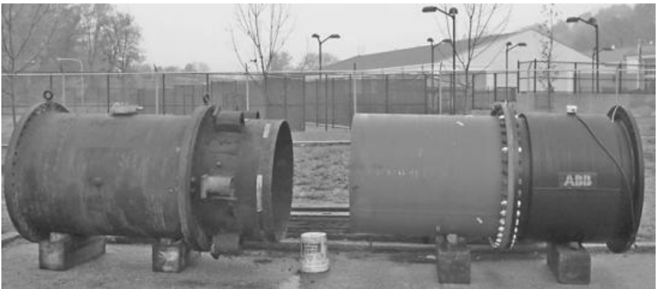
FIGURE 6.2 Source meter replacement at raw water pumping station: Existing meter removed and placed next to new 48-in diameter magnetic meter prior to its installation. (Source: Philadelphia Water Department.)
