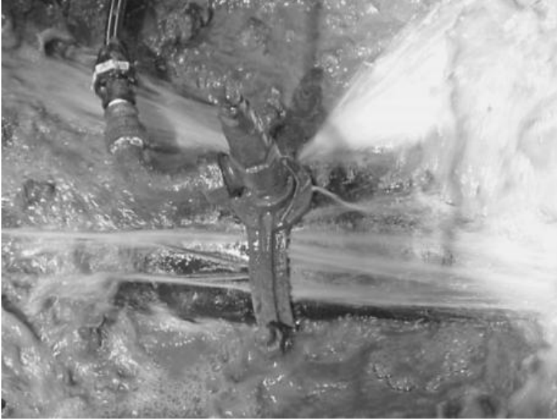
FIGURE 3.4 Service line leak. (Source: WSO—Guido Wiesenreiter.)
