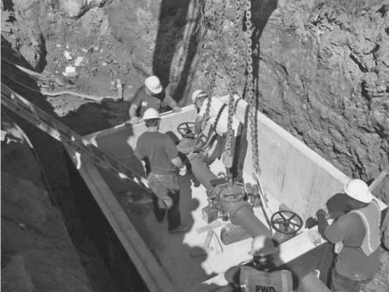
FIGURE A.1.2 Installation of pressure reducing valve and chamber for DMA5 in Philadelphia. (Source: Philadelphia Water Department.)
