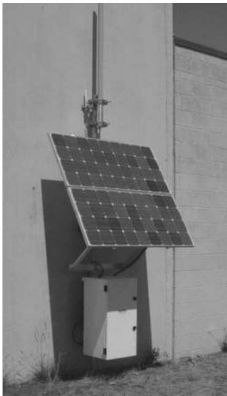
FIGURE 13.8 AMR fixed network collector antenna. (Source: Itron, Inc.)
