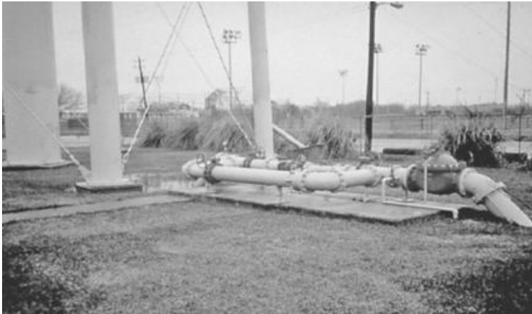
FIGURE 18.18 Altitude valve installation.
