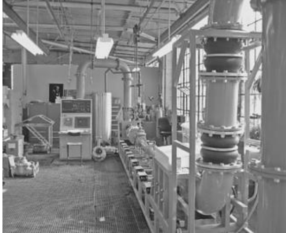
FIGURE 12.7 Water meter test bench for accuracy testing of water meters of size 3 in and larger.
