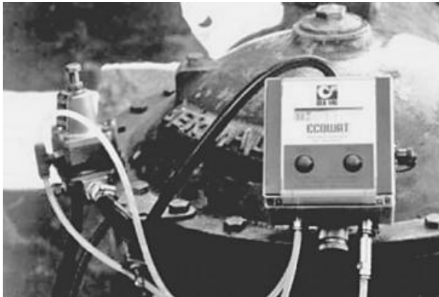
FIGURE 18.26 Time-based controller fitted to valve pilot.
