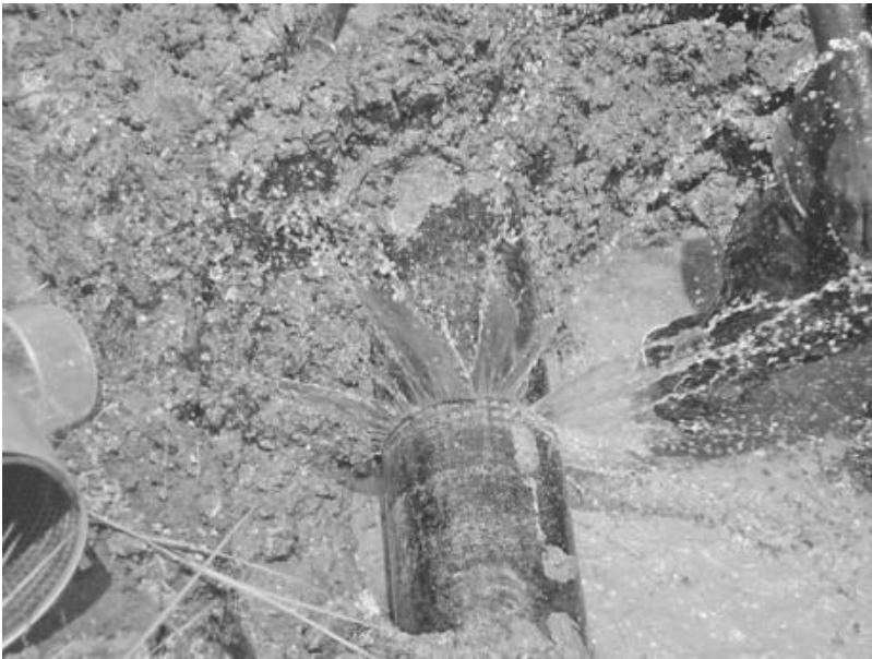
FIGURE 3.3 Distribution main break. (Source: WSO—Guido Wiesenreiter.)
