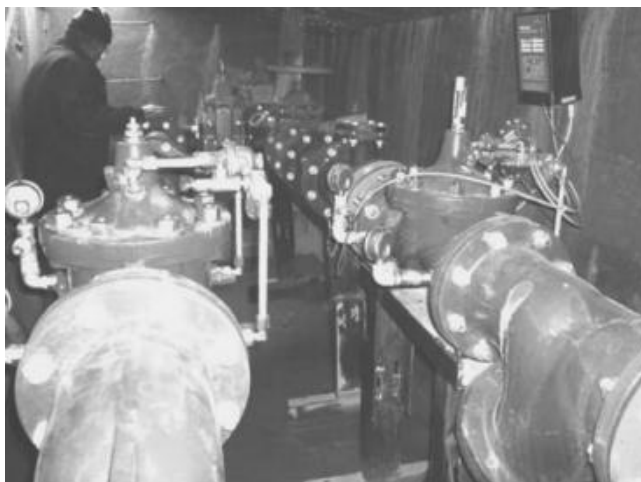
FIGURE A.15.12 Pressure control chamber. (Source: Jurica Kovac, IMGD Ltd.)
