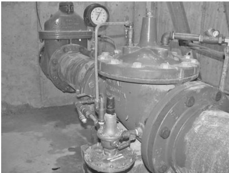
FIGURE A.1.4 Pressure reducing valve on primary supply water main for DMA5 in Philadelphia. (Source: Philadelphia Water Department.)
