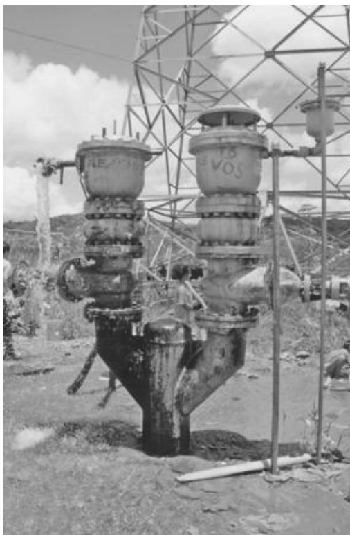
FIGURE 16.13 Visible leakage from an air valve.
