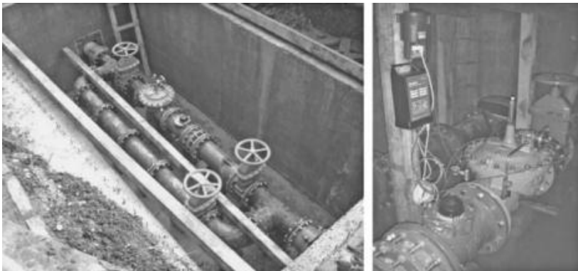
FIGURE A.15.5 Pressure control chamber. (Source: Jurica Kovac, IMGD Ltd.)
