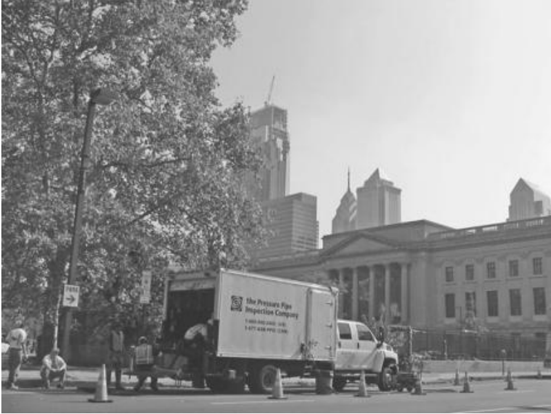
FIGURE A.1.8 Equipment setup for SAHARA inline transmission main leak detection service in Philadelphia on 48-in steel main traversing under interstate highway. (Source: Philadelphia Water Department.)
