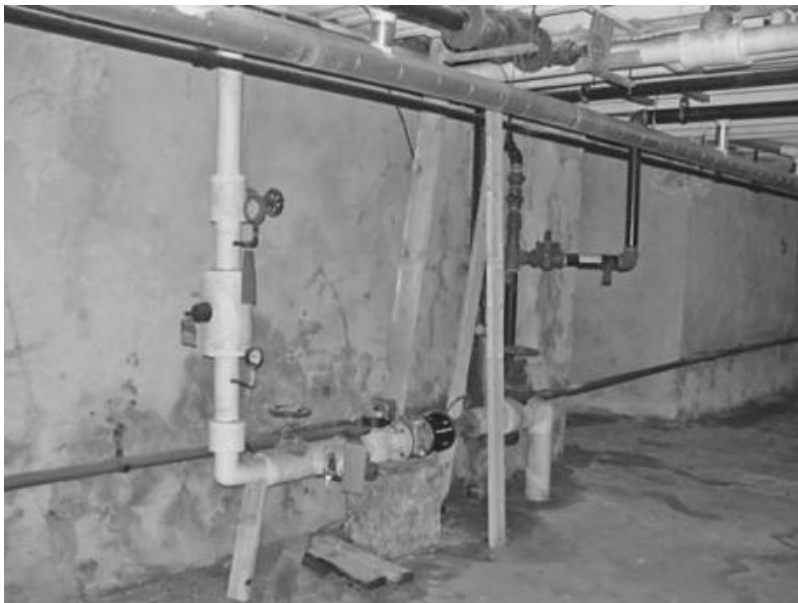
FIGURE 13.2 Indoor 3-in turbine meter servicing a 100-unit apartment building in Philadelphia showing location in underground basement of the building. (Source: Philadelphia Water Department.)
