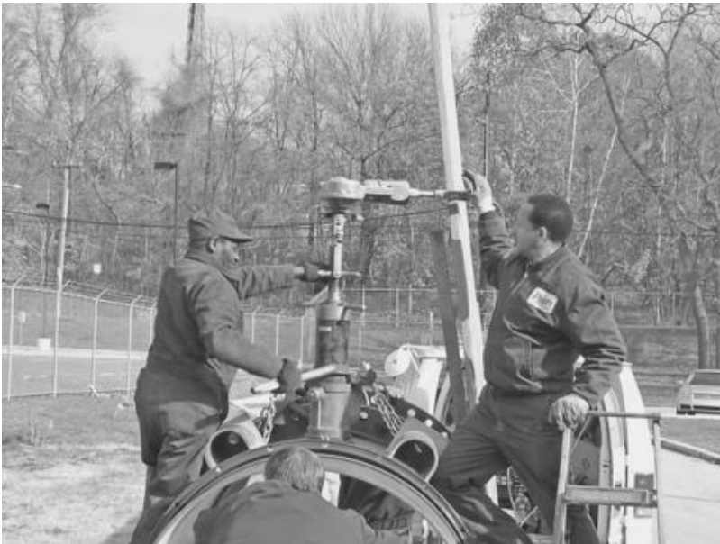
FIGURE 6.4 Source meter replacement at raw water pumping station: Ferrule being drilled into solid sleeve piping adjacent to new 48-in diameter magnetic meter. The ferrule will be used as a location for future meter verification testing by use of an insertion pitot rod. (Source: Philadelphia Water Department.)
