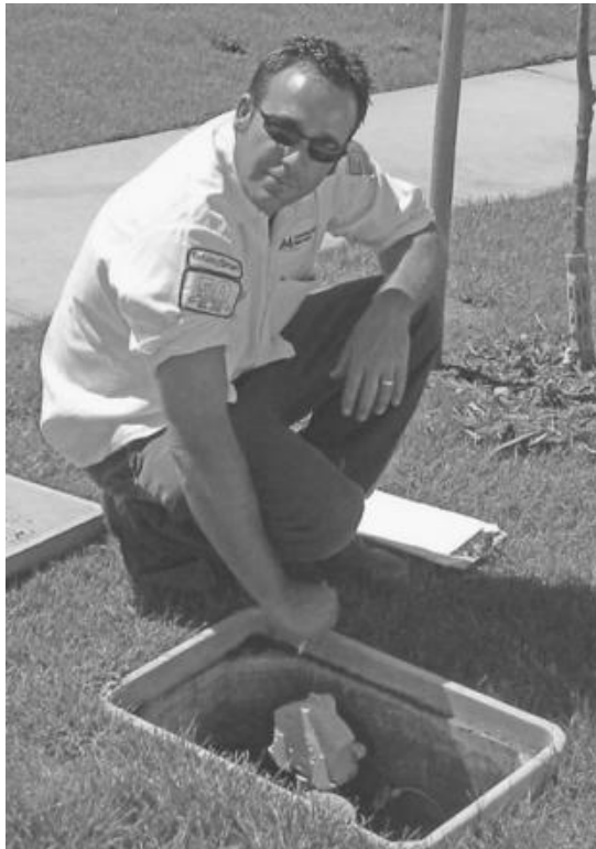
FIGURE 13.7 AMR endpoint device being installed in a residential meter pit. (Source: Itron, Inc.)
