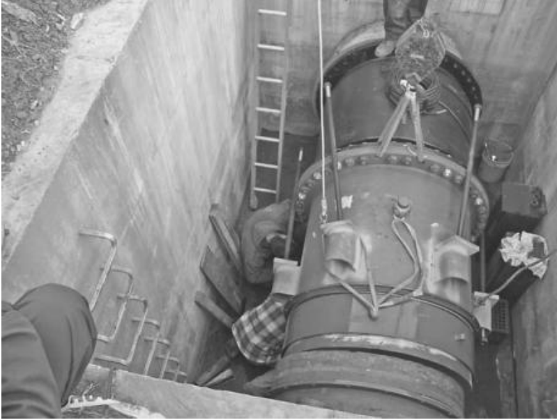
FIGURE 6.5 Source meter replacement at raw water pumping station: New 48-in diameter magnetic meter has been lowered into its chamber and work is underway to make connections to the raw water transmission piping. (Source: Philadelphia Water Department.)
