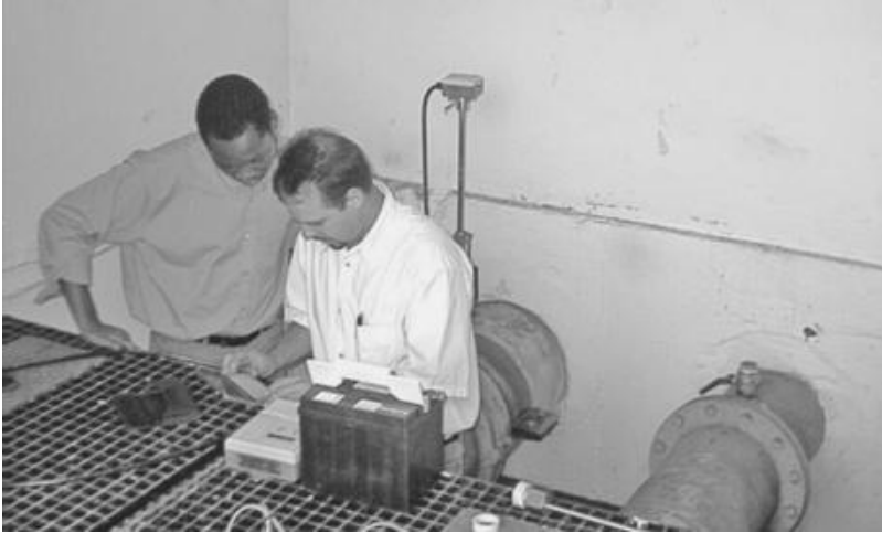
FIGURE B.3 Electromagnetic insertion meter installation. (Source: Restor Ltda.)
