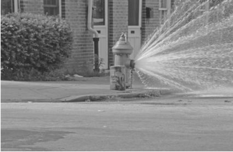
FIGURE 15.2 Unauthorized fire hydrant openings often cause damage to fire hydrants from the use of improper tools. (Source: Philadelphia Water Department.)
