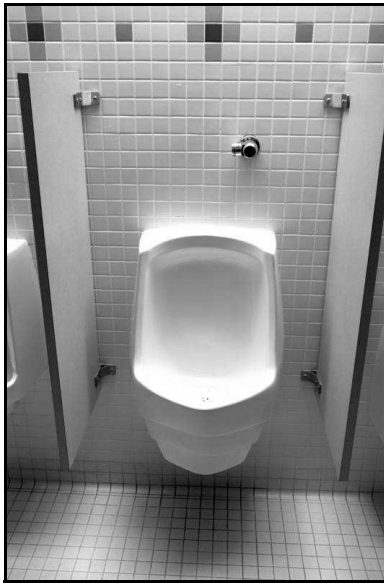
Figure 3-5 Water-saving fixture—waterless urinal
