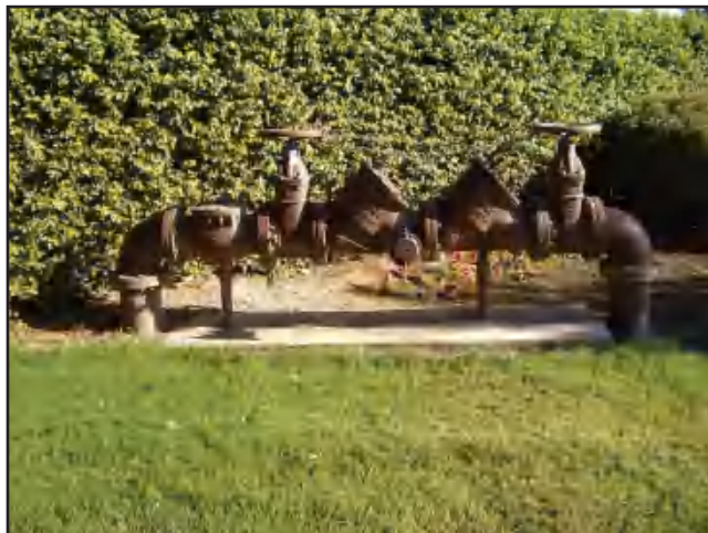
Figure A-6 Flowmeter located with insufficient spacing to allow for a streamlined flow profile and meter accuracy testing
