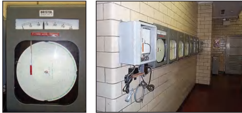
Figure A-5 Chart recorder and bank of chart recorders at the Queen Lane Pumping Station in Philadelphia, Pa.
