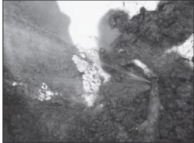
Figure 6-3 Small leak on customer service connection piping
