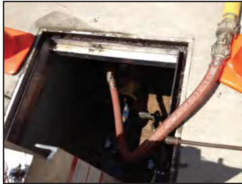
Figure 5-11 Hose connected to large meter test port in underground meter pit and ready for testing
