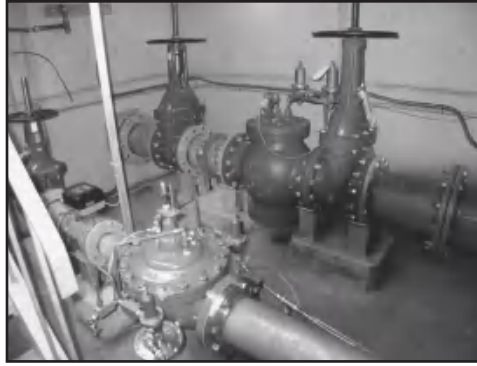
Figure 7-33 Typical pressure management and DMA supply installation
