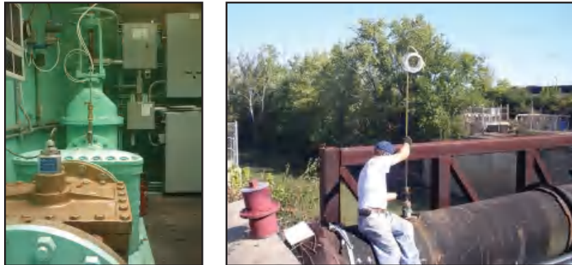
Figure A-7 Insertion Pitot rods in-place to measure flows for comparison of water flow in large flowmeters
