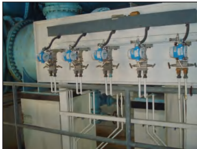
Figure A-4 Bank of differential pressure transmitters (DP cells) at the effluent pumping facility of the Crescent Hill Water Treatment Plant, Louisville, Ky.
