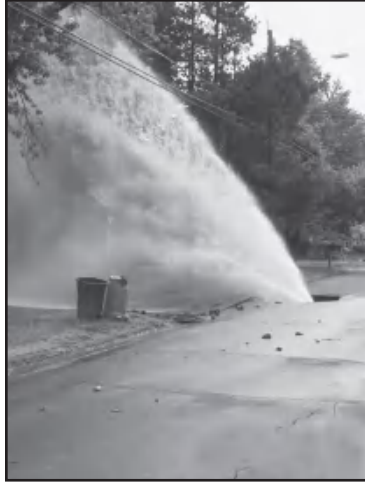
Figure 6-2 Large water main break
