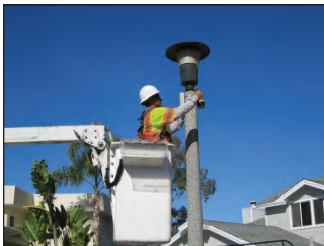
Figure 7-17 Mounting a leak detection fixed-base radio repeater on a lighting pole in the Olivenhain Municipal Water District
