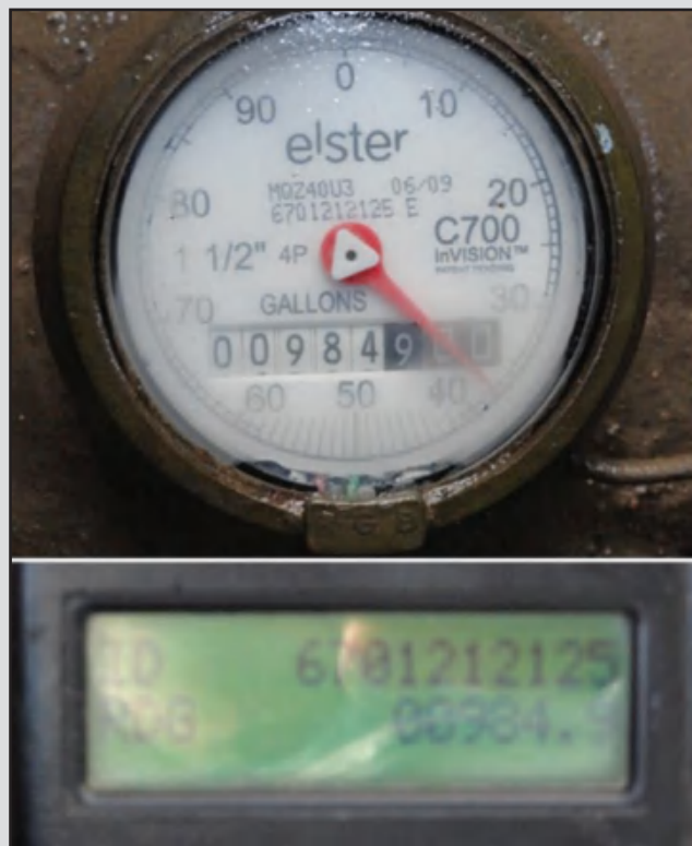
Figure 5-A Meter register showing active six digits on the meter, along with erroneous AMR touch-probe meter reading of only five digits
