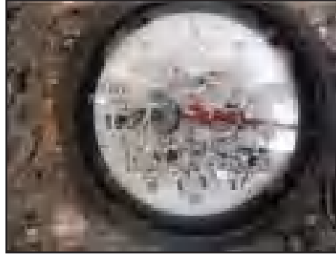
Figure 4-2 Accumulation of moisture inside a water meter register obscures the dial and prevents visual meter readings
