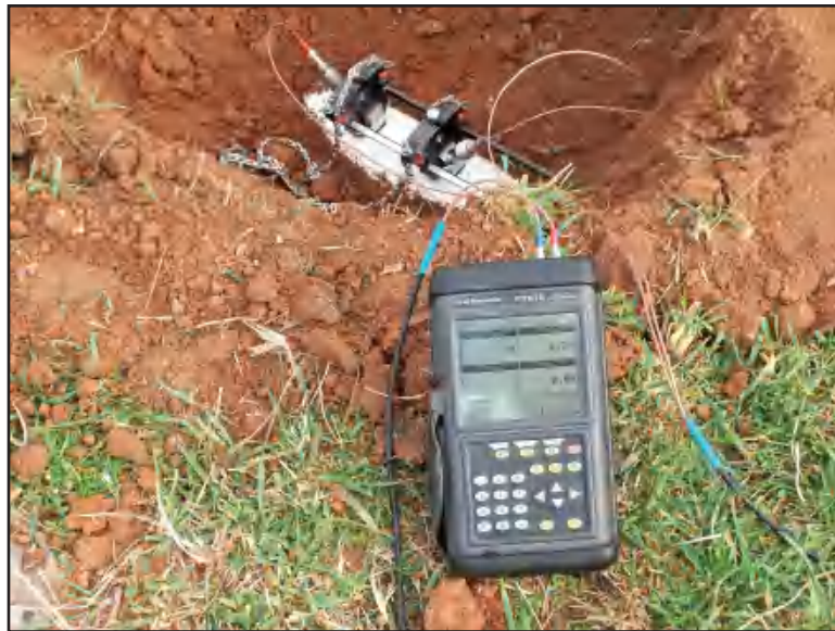
Figure 9-2 Using a portable ultrasonic flowmeter on a PVC pipeline in Wilson County, Tenn.
