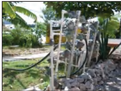
Figure 4-4 A bank of water meters showing numerous meters improperly installed at an angle instead of being properly installed upright and horizontal
