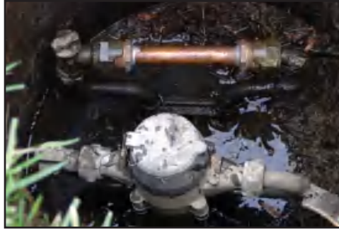
Figure 5-19 Existence of a “cheater” or “jumper” pipe (top) that was illegally used to replace the top meter in the meter setter. In the lower part of this meter pit is a typical 5/8-in. residential meter.
