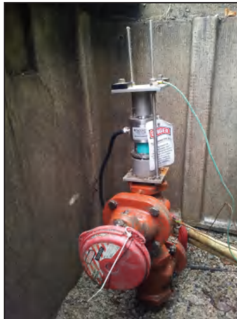
Figure A-2 Insertion magnetic flowmeter in use on a 30-in. pipeline in Birmingham, Ala.
