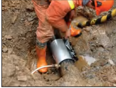
Figure 7-24 Repair clamps are commonly used to repair circumferential ruptures on distribution piping since they are quick to install and are highly durable
