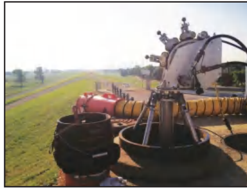
Figure 7-21 Tethered inline leak detection insertion apparatus
