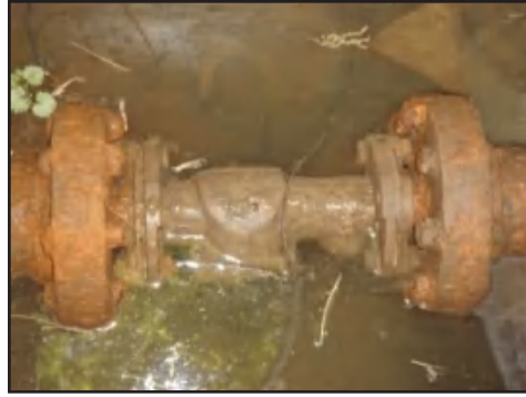
Figure 4-3 A water meter installed upside down is an example of a poorly installed meter; water meters should be installed upright and in the horizontal position
