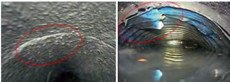
Fig. 7 Examples of corrosion/breakage
