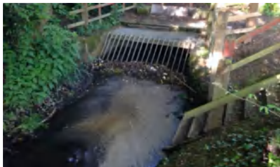
Fig. 1 Inlet trash-rack before the drainage pipe is a necessary and efficient element for catching coarse dirt taken away by water flowing down from communications and outdoor surfaces
