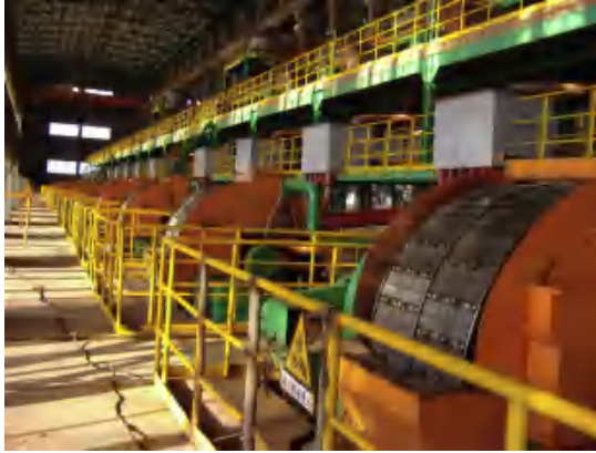
Figure 19 Operation of SLon pulsating magnetic separators in Qidashan processing plant for concentration of Anshan type lean hematite ore.
