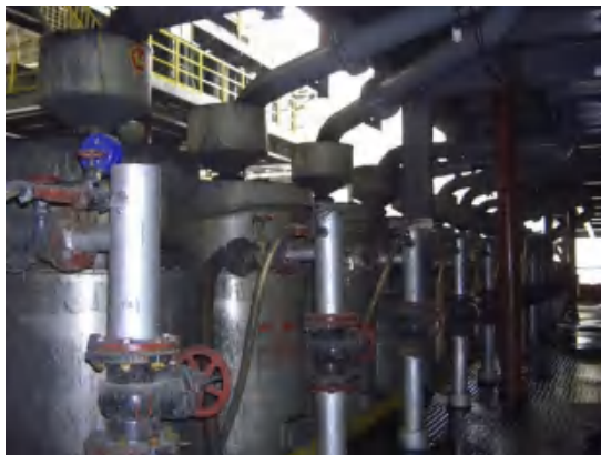
Figure 4 Operation of column magnetic separators for cleaning of magnetite.
