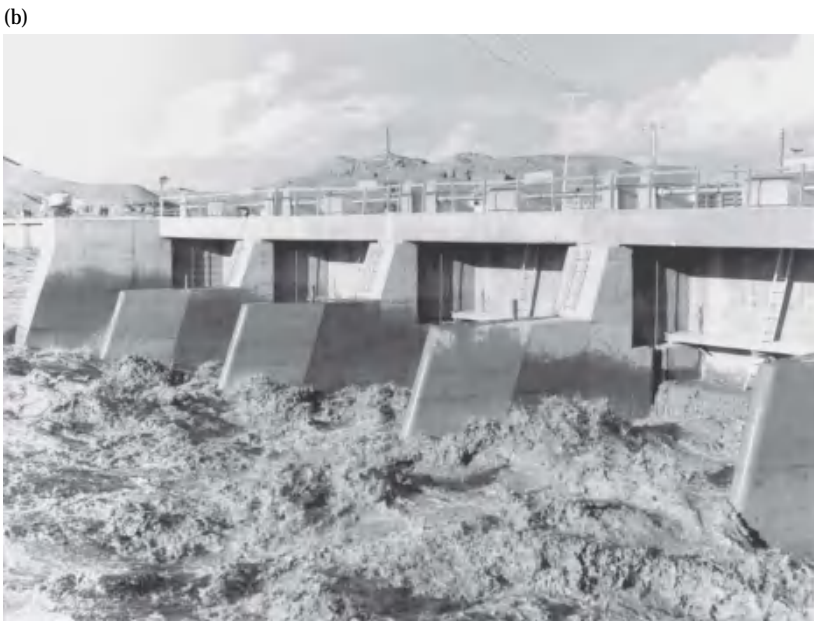
Figure 5.4 Using energy and continuity. (a) 'Free' flow under a sluice gate. (b) Sluice gates controlling discharge into irrigation canal, Iraq.
