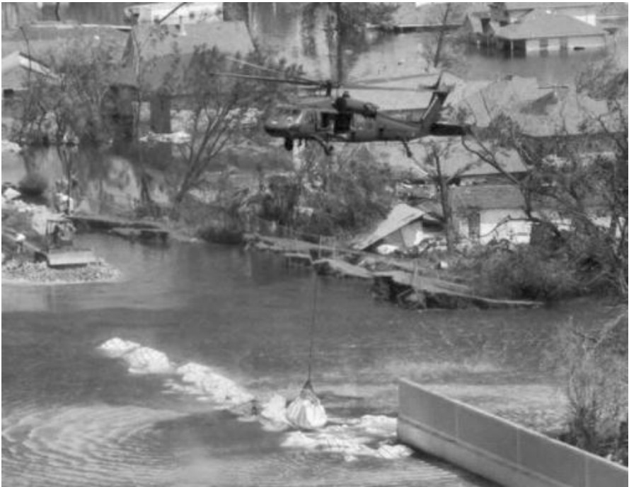
Closure of 17th Canal levee breach following Hurricane Katrina (After Seed, et al. [2005]; US Army Corps of Engineers Photograph)
