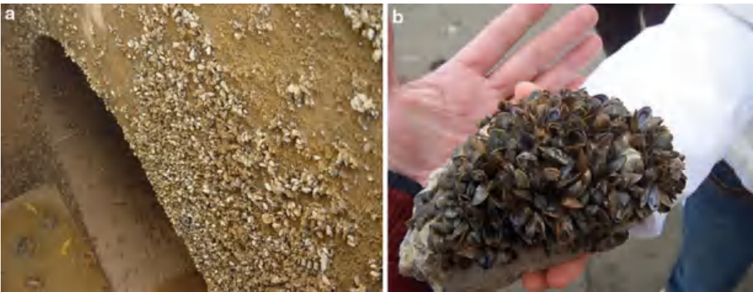
Fig. 3.23. Colonization of golden mussel on concrete walls in a water transfer tunnel and attachment of golden mussel on a concrete fragment with high density.
