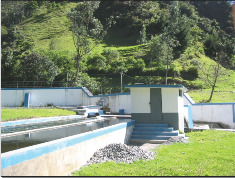
View of the sedimentation of the catchment of water in the El Carmen creek
