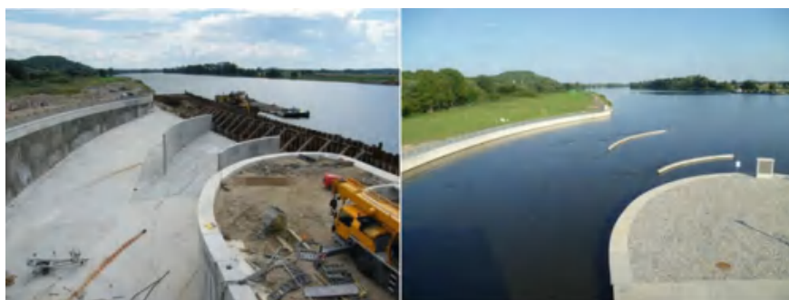
Fig. 15.8 Intake part of the SHPP Litoměřice under construction (left) and after completion (right)
