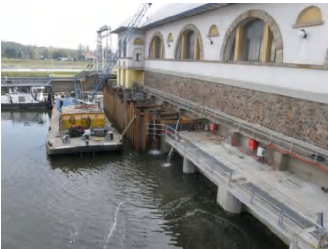
Fig. 15.18 Construction works on the outlet part of the SHPP including modification of the draft tubes of turbines and installing new draft tube stop logs
