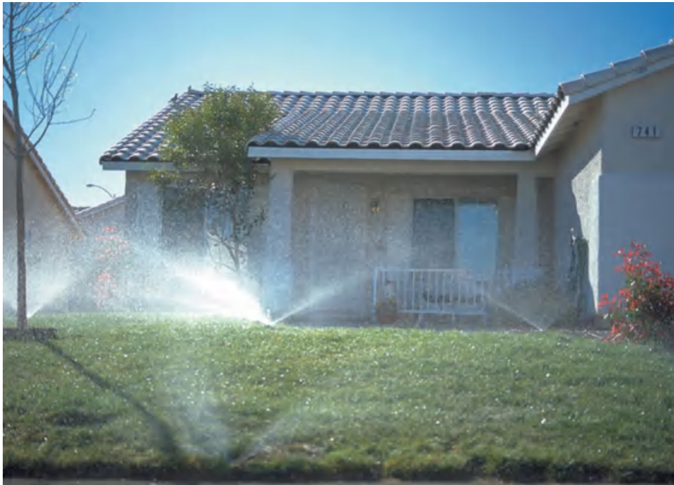
Fig. 1.9 Turf irrigation system (Credit NRCS)
