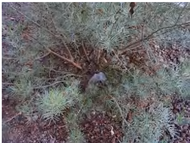
Fig. 15.9 Bubbler at base of shrub
