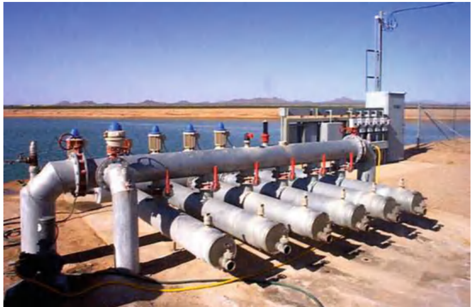
Fig. 12.30 Reservoir and pump station for center pivot farm. Cylindrical stainless steel ring filters and manifold in foreground. Motors on top of turbine pumps are seen behind manifold (Credit Paul Colaizzi, University of Arizona and USDA-ARS Bushland, Texas)
