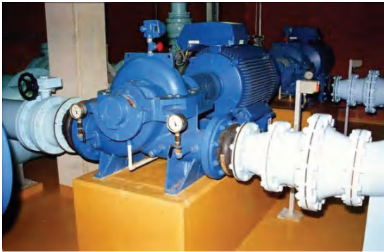
Figure 4.120 Horizontal pumps with rubber rings to dampen vibration
