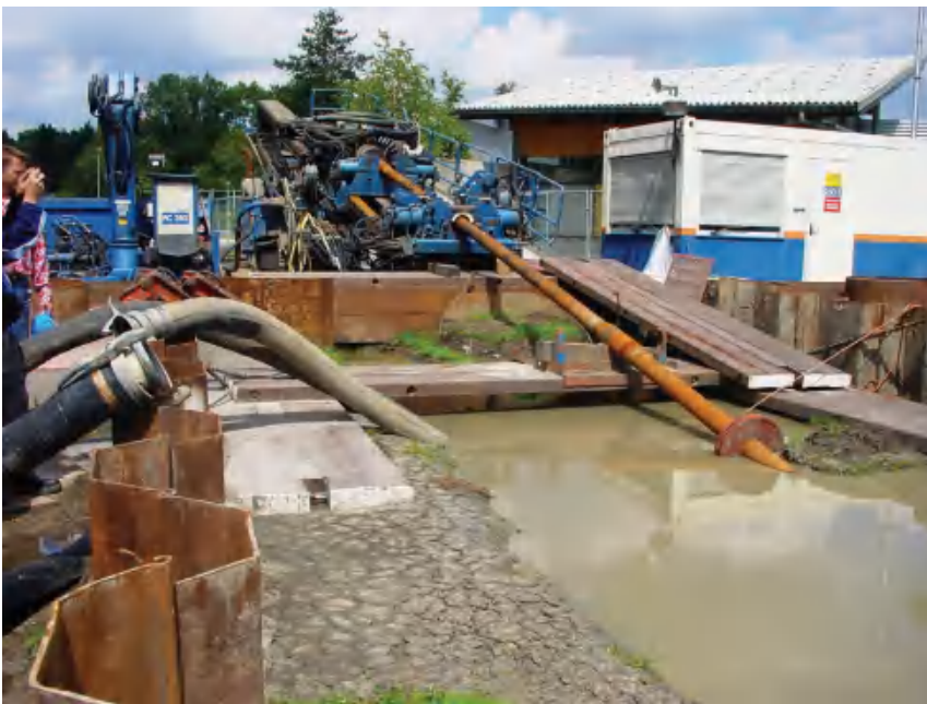
Figure 5.15 Boring in friable soils, upstream view
