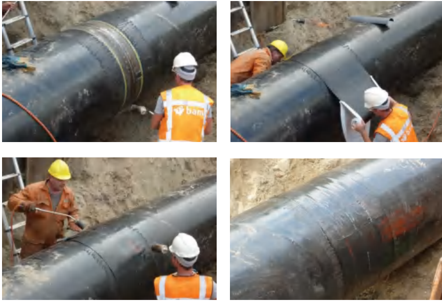
Figure 4.60 An alternative method of protecting the steel joint by melting the PE tape
