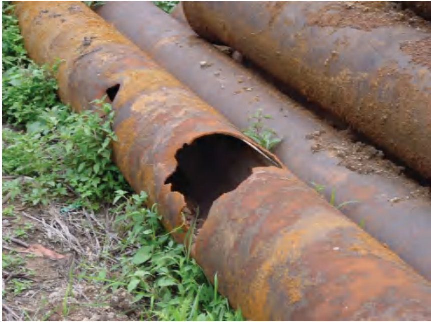
Figure 6.31 Damaged steel pipes taken out of operation.
