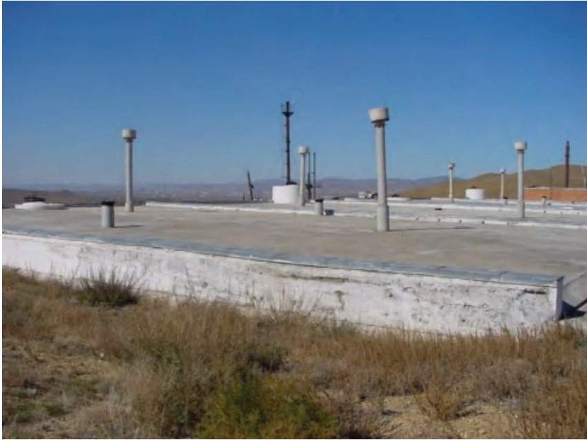
Figure 4.113 Protected air vents on an underground reservoir
