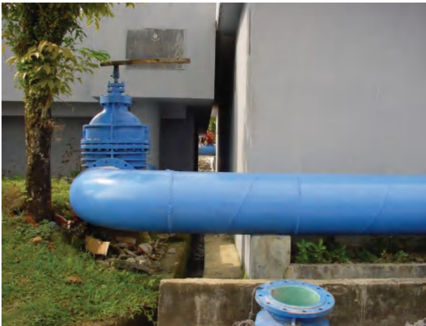
Figure 4.41 A spirally-welded steel pipe protected with anticorrosive paint
