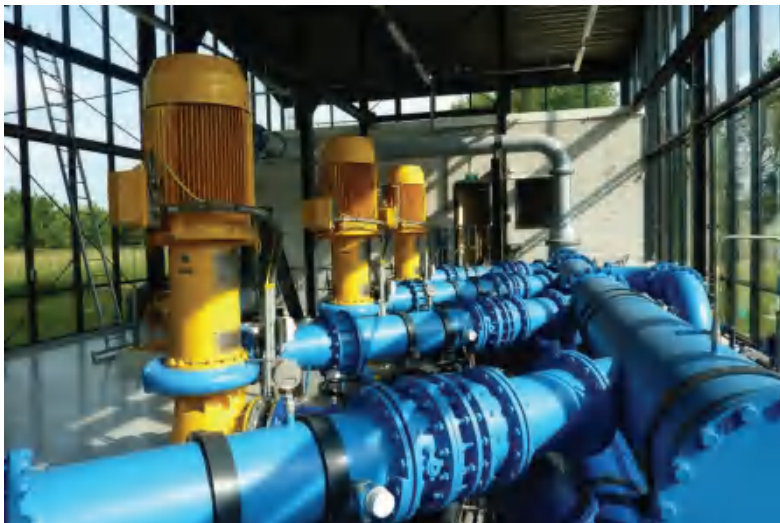
Figure 4.121 An unmanned booster pumping station
