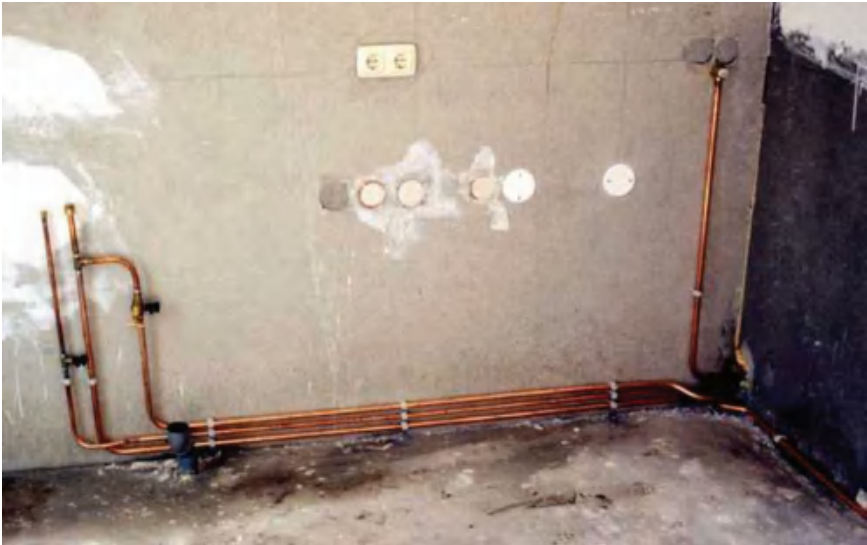
Figure 4.45 Indoor installations made of copper
