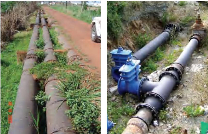
Figure 4.3 Parallel water transportation pipes
