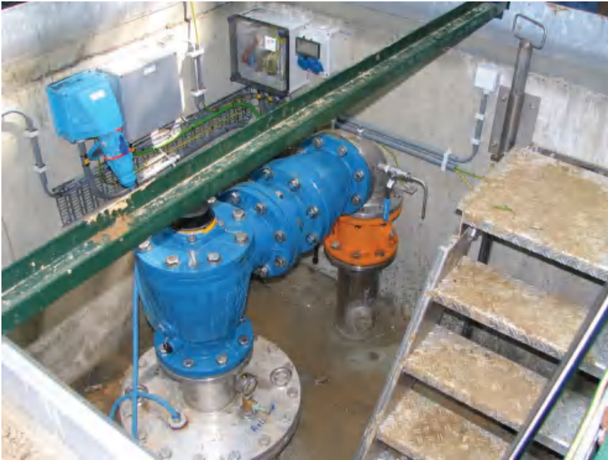
Figure 1.18 Deep well pump at the groundwater source
