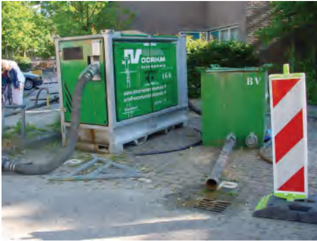
Figure 5.22 A lateral pipe connected to the pump and the discharge box to the sewer
