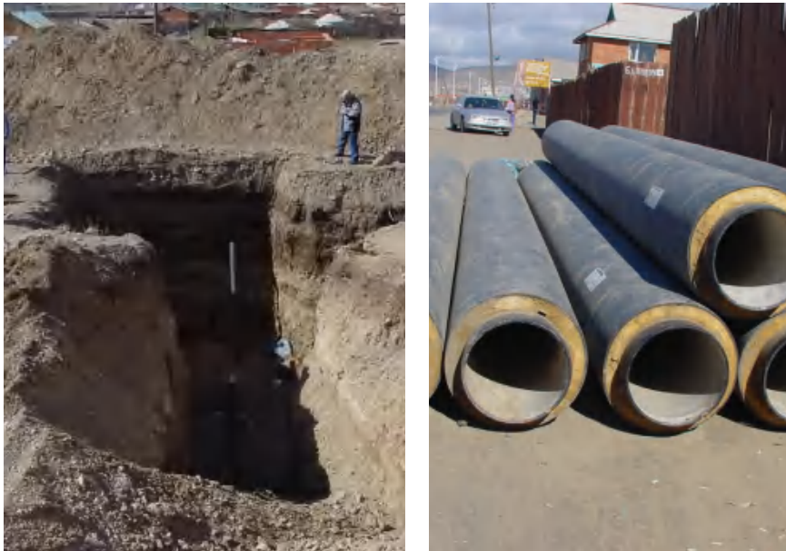
Figure 5.14 Trench depth (left-hand side) and insulated DI pipes (right-hand side) in Ulaanbaatar, Mongolia
