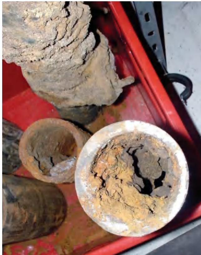
Figure 4.36 Heavily corroded cast iron pipes
