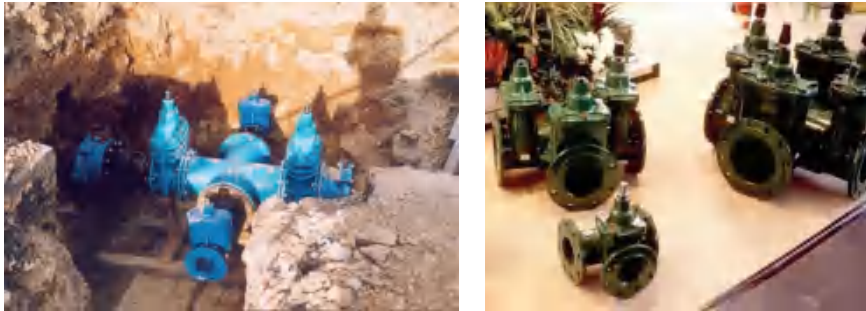
Figure 4.74. Blocks of gate valves.
