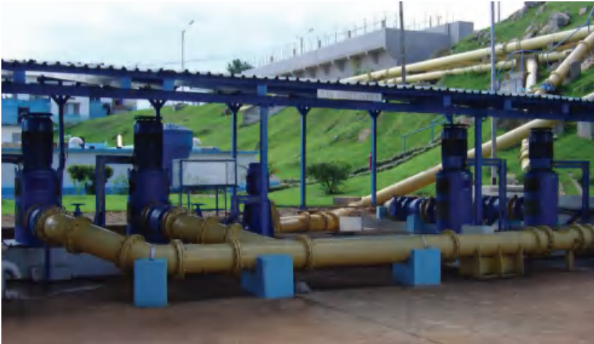
Figure 5.32 Steel pipes clamped on a concrete support and protected by a roof
