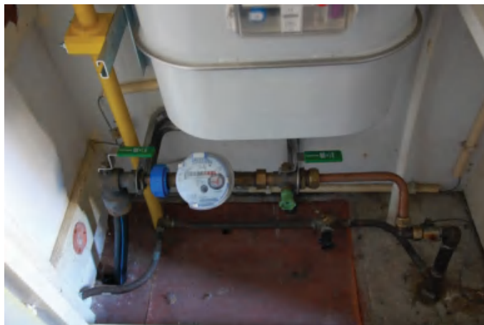
Figure 4.110 Indoor metering set-up connected to the PE service pipe (on the left)
