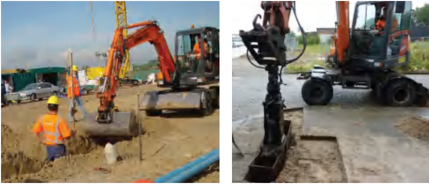
Figure 5.6 Mechanical excavation in sand: a wide trench (left-hand side) and a narrow trench (right-hand side)
