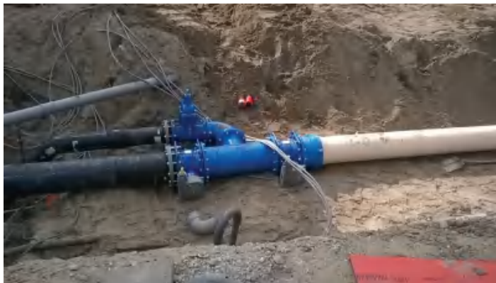
Figure 4.70 Connection of PE and PVC pipes to a valve block made of DI
