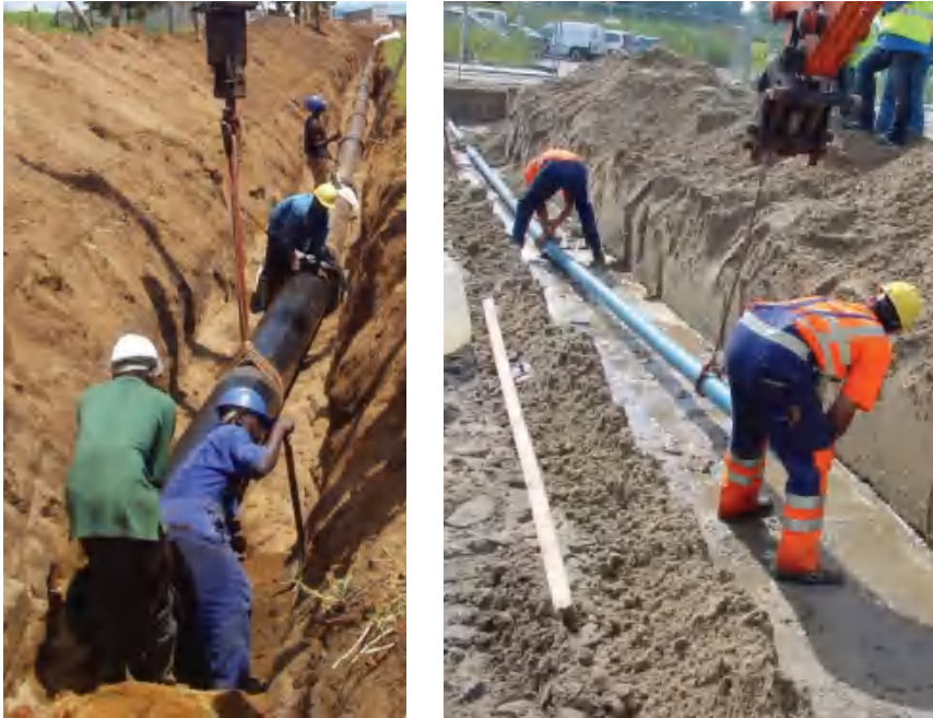
Figure 4.40 Laying of DI pipes (large diameter – left-hand side, small diameter – right-hand side)
