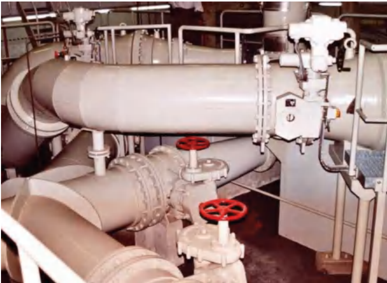
Figure 4.119 Piping in a pumping station
