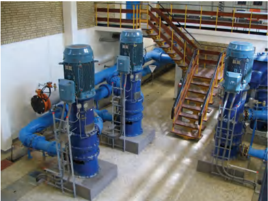
Figure 1.21 Vertical centrifugal pumps with frequency controllers for variable speed
