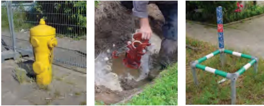
Figure 4.101 A ground-level fire hydrant (left-hand side), underground fire hydrant (centre) and sign post (right-hand side)
