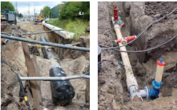
Figure 5.1 Pipe laying: a transportation steel pipe (left-hand side); a distribution PVC pipe (right-hand side)
