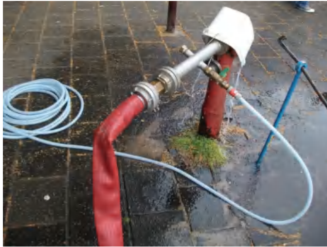
Figure 4.106 Water quality sampling using hydrants
