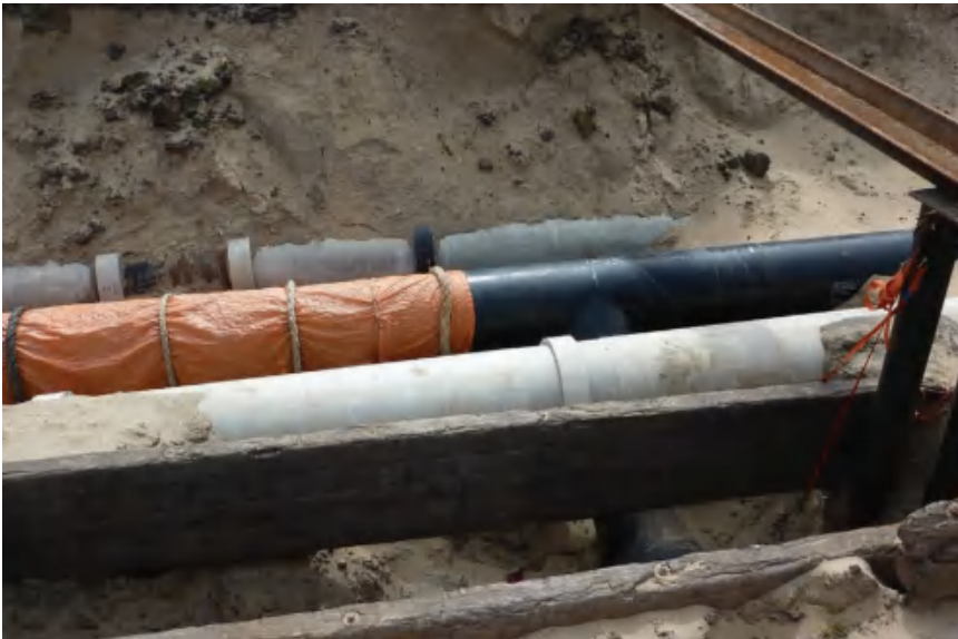
Figure 4.48 Two AC pipes parallel to the coated steel pipe (in the middle)
