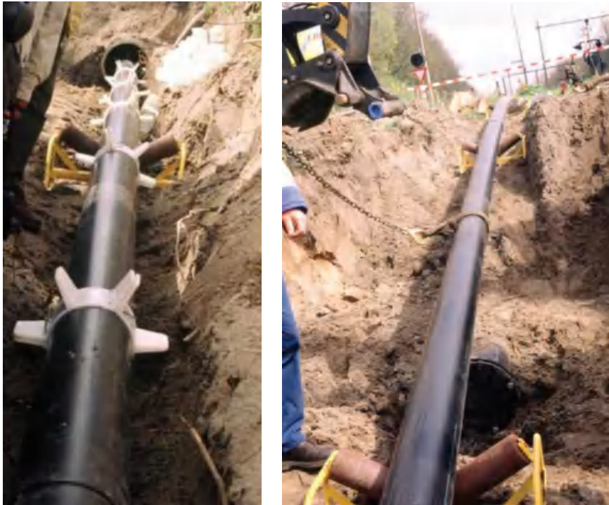
Figure 5.31 Casing of a PE pipe in an old CI pipe (left-hand side); the opposite view (right-hand side)
