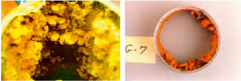
FIGURE 2 The interior of many distribution system pipes can present a very hostile environment for sensor deployment. Photos courtesy—US Army Corps of Engineers (see Plate 4 of Color Plate section).
