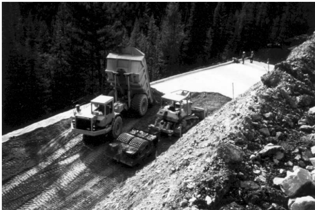
FIGURE 37.6 Placement of a high-strength nonwoven geotextile to perform a dual function of reinforcement and in-plane drainage in a reinforced slope.
