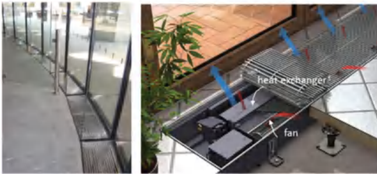
Fig. 8.19 Convectors installed into the floor below glass façade to compensate a cold air jet that descends from the glassing; draught is eliminated and thermal comfort is improved (left); (Bridge & PR Media Service Ltd.) forced convection fan-coil convector installed in a raised floor (right) (KI TDC d.o.o.)
