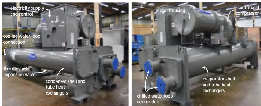
Fig. 9.14 Water-cooled vapour compressor refrigeration machine or chiller, full cooling capacity 123 MW c (350 ton), motor electrical power 250 kW e , rated COP 4.933 (Carrier, Evergreen 19 XR, Hermetic centrifugal water chiller)
