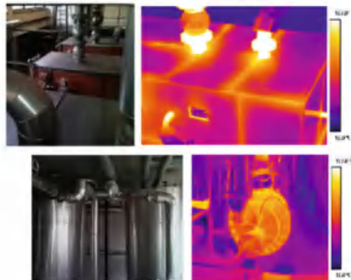
Fig. 4.12 Thermal images of case study building envelope and building service system elements
