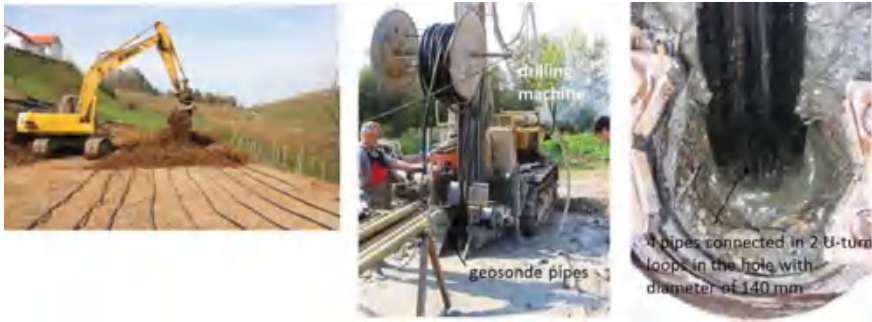
Fig. 6.19 Horizontal soil heat exchanger (left), vertical heat exchangers are up to 100 m deep and are called “geosondes” (right)
