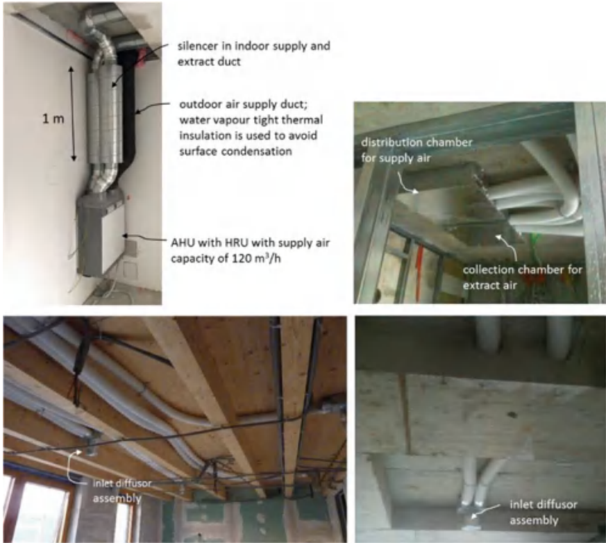
Fig. 11.27 Octopus type of distribution duct system in apartment; each tube has diameter of 80 mm and air flow rate is designed to 30–40 m 3 /h per duct; this corresponds to the physiological needs of one person. If two persons are expected to be in the room, two ducts are connected to the assembly of inlet diffuser
