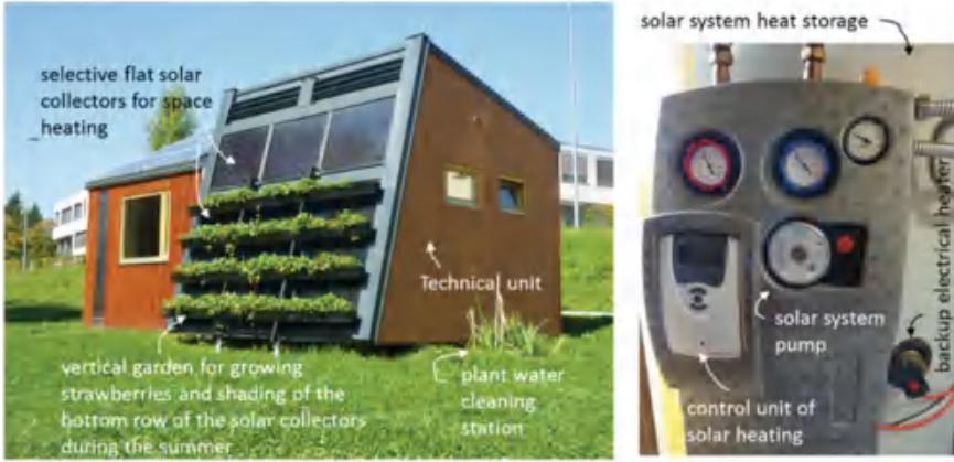
Fig. 8.41 Solar thermal collectors and heat storage of solar space heating system
