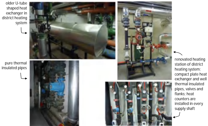
Fig. 8.45 Renovation of district heating station decrease heat consumption in multi-family buildings up to 20%
