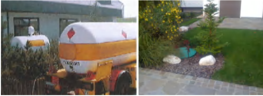
Fig. 2.17 Transportation of LPG. LPG is stored in the external or underground reservoirs. Environment heat is used for the evaporation of LPG into gas before entering the distribution pipeline in building
