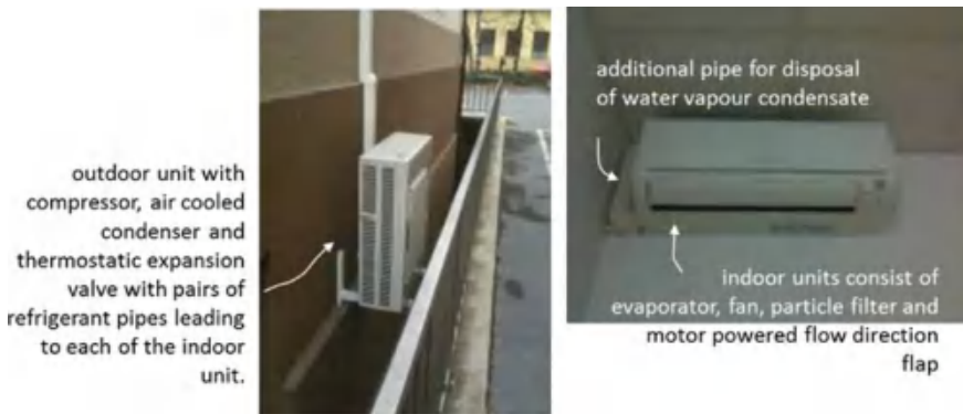
Fig. 9.12 Multi-split DX space cooling system in renovated office building
