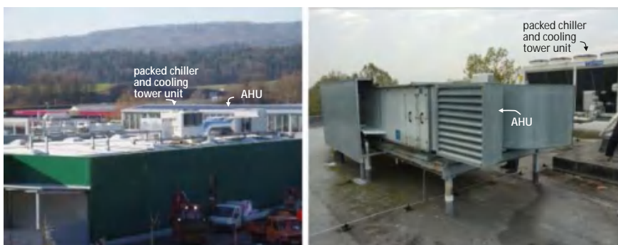
Fig. 9.15 Packed chiller and cooling tower unit on the top of the roof of shopping centre (left) and office building (right). To prevent freezing of water in the outdoor section of a chilled water loop (i) antifreeze fluid (glycol) could be added to chilled water, (ii) pipeline could be heated by a wire electrical resistance heater installed on the pipes’ outer surface, (iii) a chilled water pipeline can be drained manually until next cooling season
