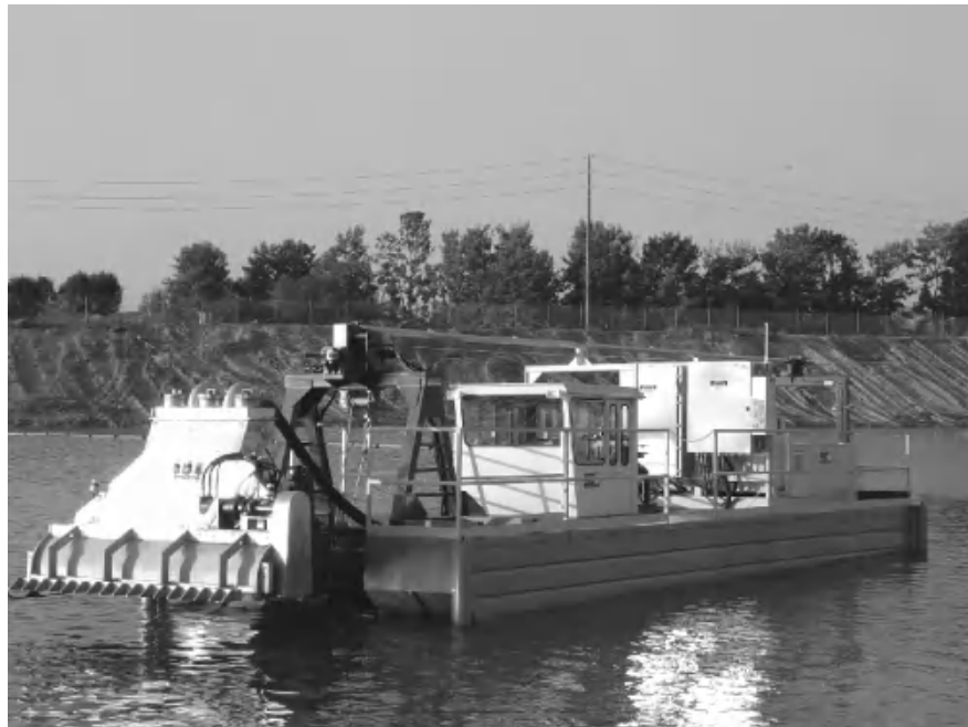
FIGURE 6-5 Basin cleaning vehicle (BCV) developed by Orange County Water District, California. This type of system allows clogging material to be removed while avoiding the water loss and expense associated with the downtime for draining and cleaning basins. Photo courtesy of Greg Woodside, Orange County Water District.
