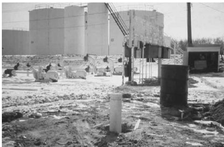
FIGURE 2.89 Above-ground storage tanks and the associated transmission pipelines and distribution piping were the focus of this investigation, during which a combination monitoring and recovery well (foreground) was installed.
