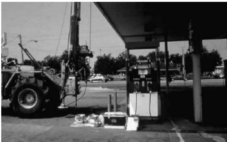
FIGURE 2.71 Other obstacles to the field investigation include canopies, pump islands, underground product distribution lines, and rebar-reinforced concrete depicted here.
