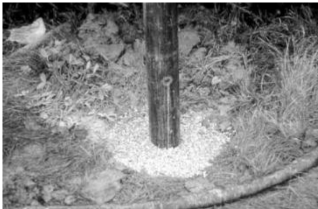
FIGURE 10.127 In cold climates, a bentonite pellet or chip surface seal may be a better choice than cement or concrete.
