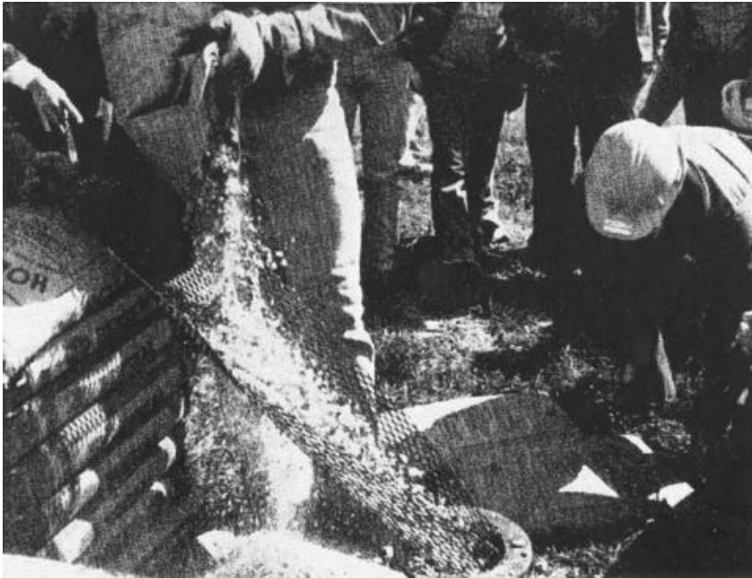
FIGURE 12.4 Filling a large-diameter well with chip bentonite. Bentonite is being poured over 1/4-in. mesh to separate the fines.
