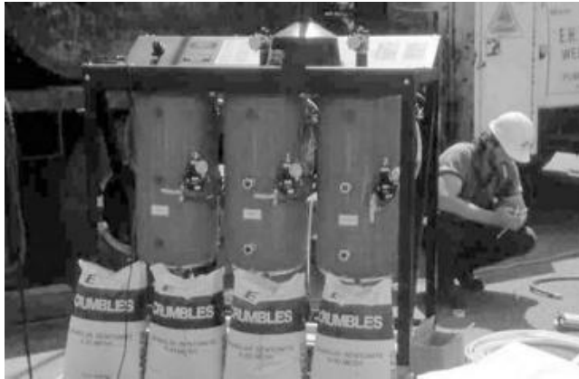
FIGURE 10.118 A dry injection system for the placement of annular seal (and filter-pack) materials in monitoring wells.
