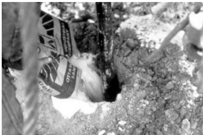
FIGURE 10.86 Placement of filter-pack sand by pouring down the annular space should only be attempted in wells less than 20-ft deep installed in relatively cohesive formations that will not collapse into the borehole during placement.
