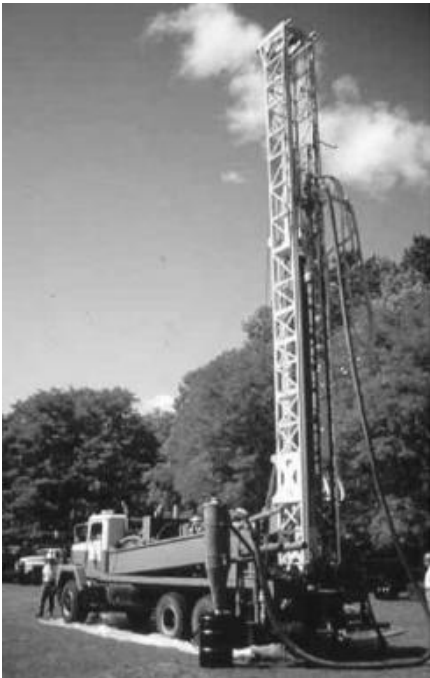
FIGURE 10.38 Dual-tube reverse-circulation rotary drilling is a useful method to overcome difficult drilling conditions, including cavernous or highly fractured bedrock and bouldery unconsolidated materials.
