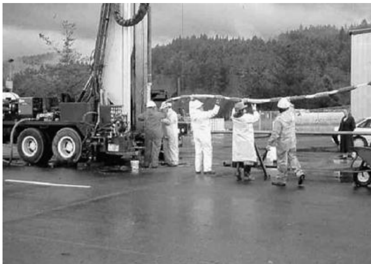
FIGURE 2.114 Sonic drilling rigs can rapidly advance boreholes through most types of geological materials and can provide for installation of long-term monitoring wells and multilevel monitoring systems. Installation of a seven-channel CMT system is shown here. (Photo courtesy of Murray Einarson.)
