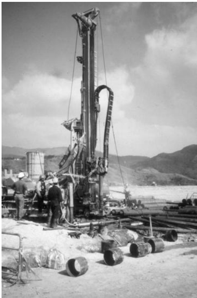
FIGURE 19.2 A cluttered site is an unsafe site.
