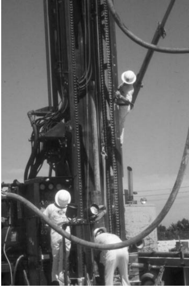
FIGURE 19.7 Fall protection is an important consideration.
