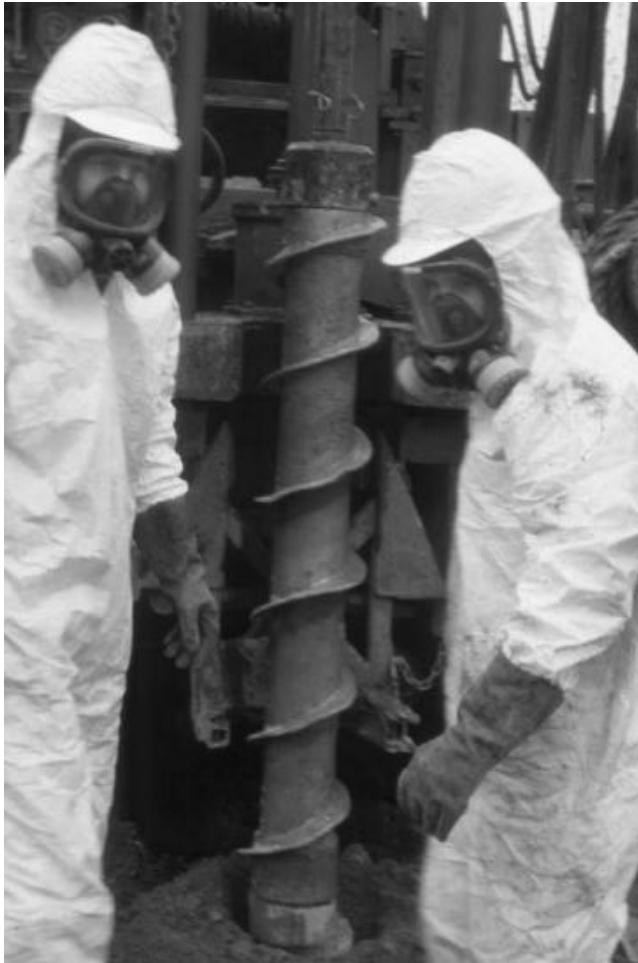
FIGURE 19.3 PPE must be carefully selected after considering the types of contaminants present and the engineering controls.
