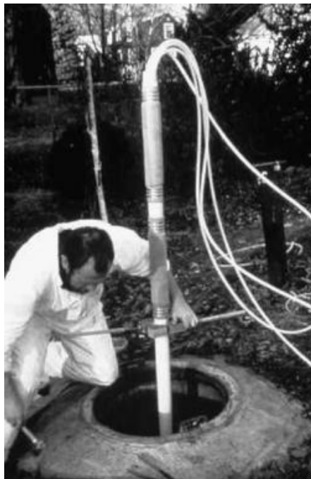
FIGURE 10.31 Installation of a multilevel monitoring system in a bedrock borehole. (Photo courtesy of Westbay Systems Inc.)
