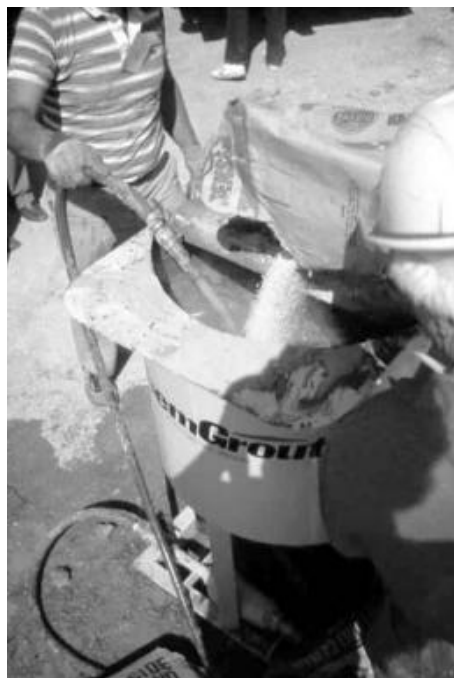
FIGURE 10.119 Granular bentonite may be mixed with water and an organic polymer (to retard hydration) into a grout that can be tremied into the borehole.
