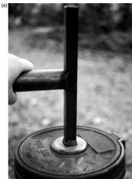
FIGURE 10.148 A special tool is required to open this lockable well vault. This sequence of three photos (a–c) shows the steps necessary to access the well.
