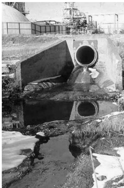
FIGURE 2.3 Industrial discharges to surface-water systems have been regulated by the Clean Water Act since 1970. Despite this, some unpermitted discharges still occur. These discharges can contaminate surface water and ground water, through leakage in the sewer line between the point of origin and the discharge point.
