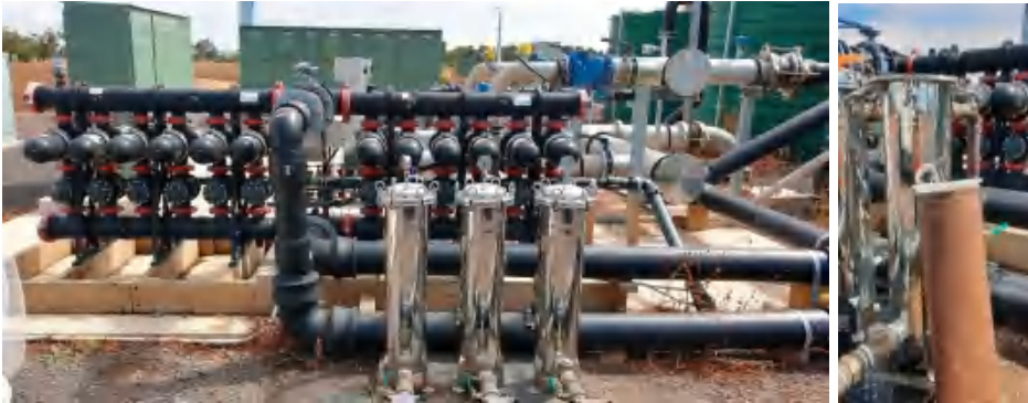
Figure 8. (Left): Central manifold ASR System with temporary prefiltration unit that includes a 20 \mu\text{m} spin Klin disc (the 12 black cylinders) followed by a 1 \mu\text{m} bag filter (the 3 upright cylinders). (Right): clogging of the 1 \mu\text{m} bag filter after \sim 2 days of operation.
