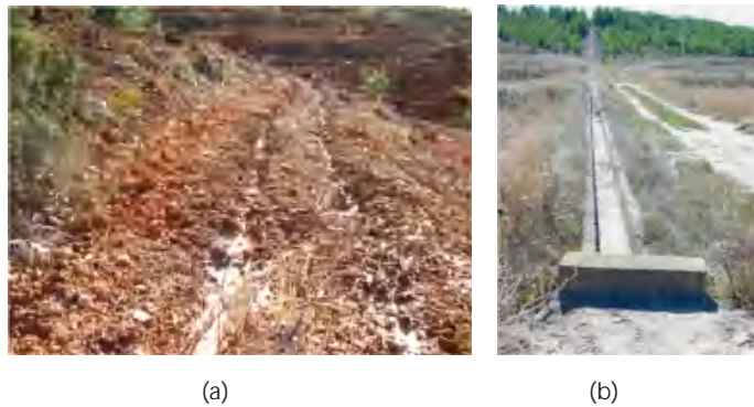
Figure 10. Mechanical initiatives to minimise runoff, facilitate recharge, and subsequent plantation (a) and infrastructure to channel and level excess runoff water (b) Neila (Castilla y León).
