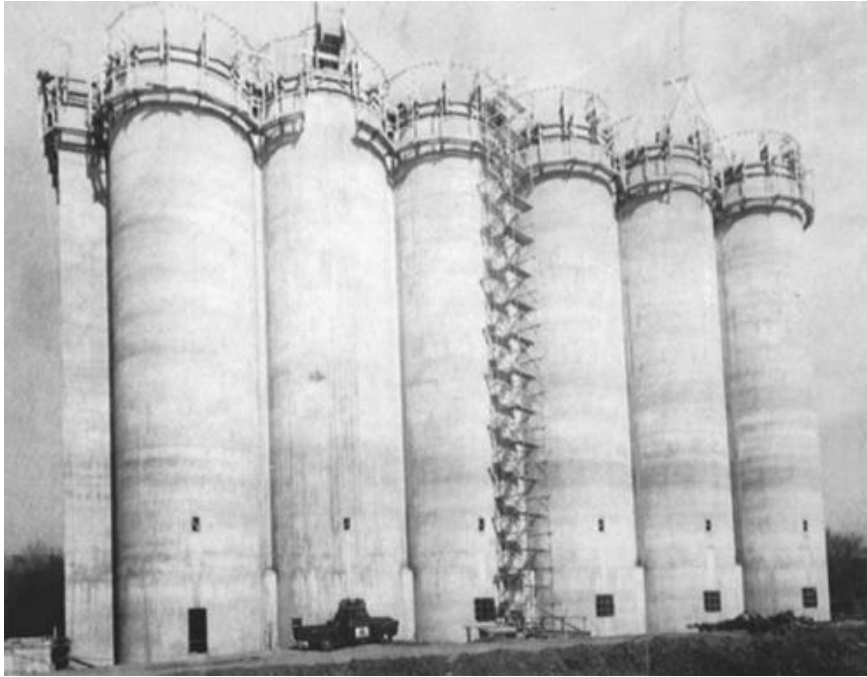
FIGURE 5.7 Trouble-saver sectional scaffolding with built-in step units for silo access during construction. Similar installations are quickly erected for many industrial maintenance operations when the safe, speedy vertical movement of persons is needed. ( The Patent Scaffolding Co., Inc. Photo by Tracy O'Neal. )
