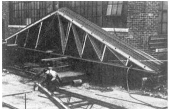
FIGURE 1.5 Maintenance department fabricating trusses for plant expansion. Trusses made from channels and angles. A jig was laid out on plate in the plant yard.
