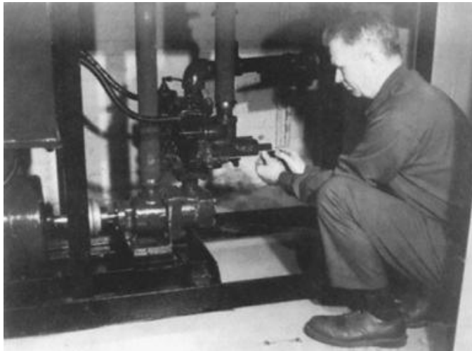
FIGURE 4.3 Oil-hydraulic elevators for freight or passenger service receive the attention of the manufacturer’s maintenance specialists skilled in servicing the inter-related electrical, hydraulic, and mechanical subsystems that must function efficiently in unison for the elevator to provide quiet, dependable service. Valve adjustment is one of many conditions that must be checked with a high degree of accuracy.
