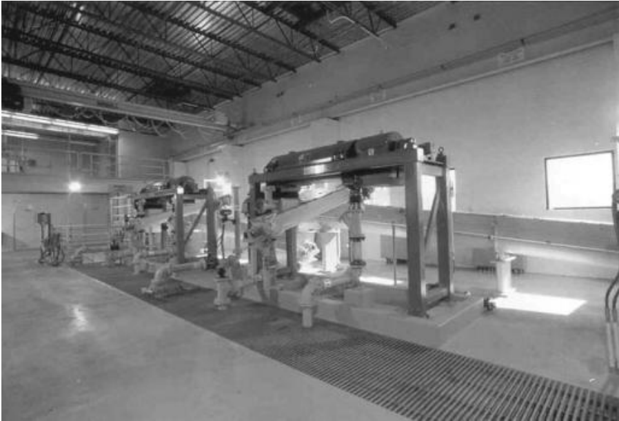
Fig. 23–14. Solid bowl centrifuges at Verde Water Treatment Plant (Courtesy of City of Phoenix and Alfa Laval Inc., Warminster, PA)
