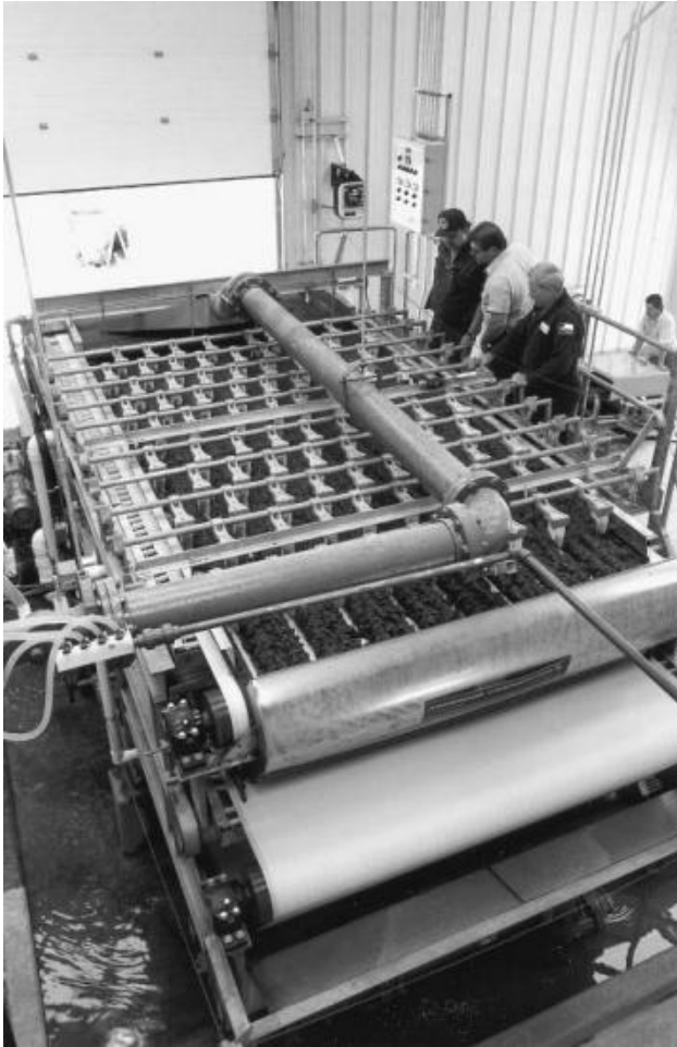
Fig. 23–17. Belt press installation at Cedar Park, Texas, water-treatment plant (Courtesy of Ashbrook-Simon-Hartley)
