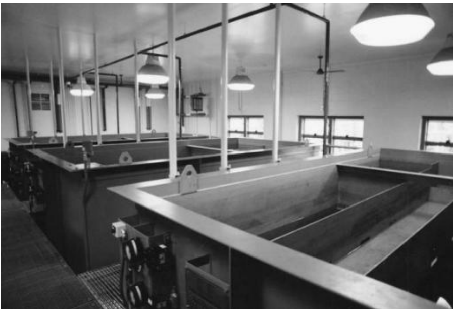
Fig. 25-13. Photo of Advent package plant (Courtesy of Infilco Degremont, Inc.)
