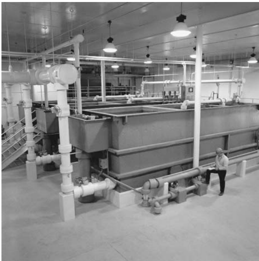
Fig. 25-11. Photo of 700-gpm Pacer II package plant (Courtesy of Roberts Water Technologies)
