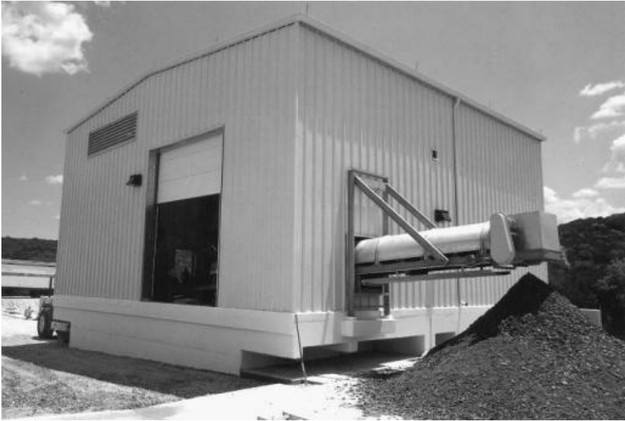
Fig. 23–18. Alum sludge cake discharging from belt filter press at Cedar Park, Texas (Courtesy of Ashbrook-Simon-Hartley)
