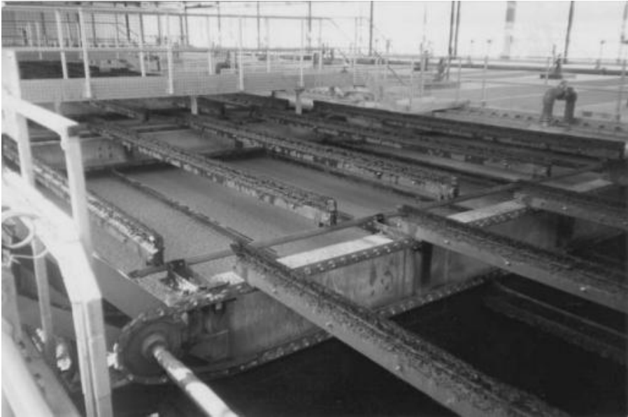
Fig. 11–27. Dissolved air flotation system at the Arvika Water Treatment Plant in Sweden (Courtesy of The F. B. Leopold Company Inc.)
