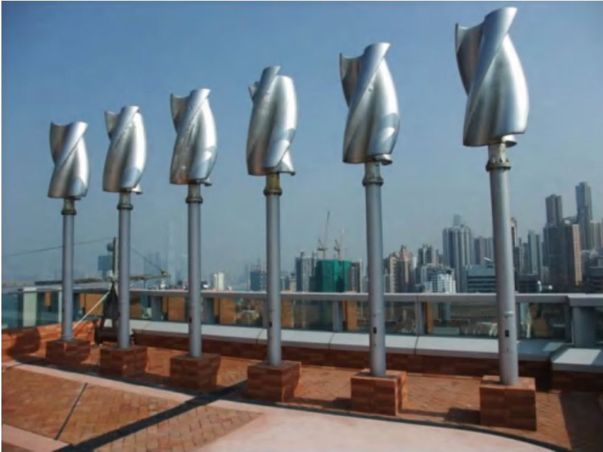
Fig. 7.4 Photo of vertical axis wind turbines installed on top of a building at the Hong Kong University campus
