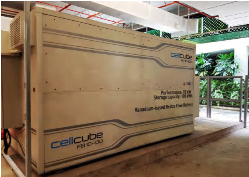
Fig. 7.6 Photo of a Vanadium Redox-flow battery (VRB) installed in the basement of building in Singapore
