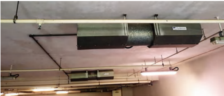
Fig. 5.10 Photo of ductless jet fans installed in a car park of a building in Singapore
