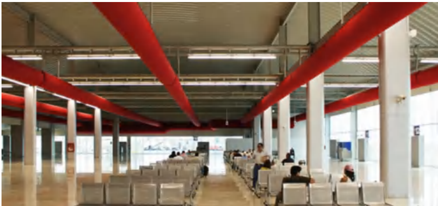
Fig. 5.9 Photo of a site with fabric duct installed (DuctSox.com)
