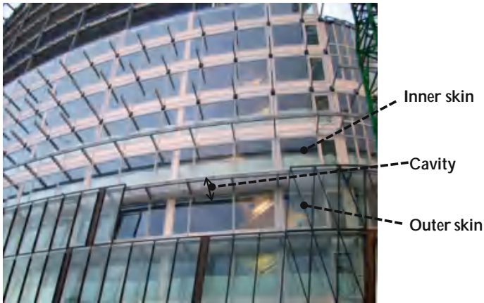
Fig. 4.18 Photo of a building in London showing a double-skin facade being assembled
