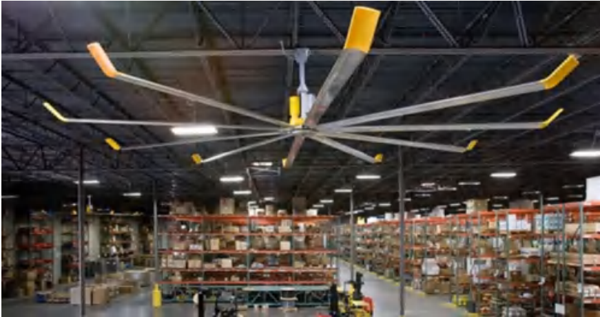
Fig. 5.11 Photo of HVLS fan installed in an industrial workshop space (Kestrel Services)
