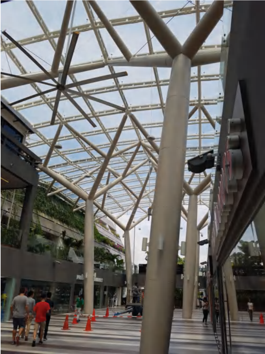
Fig. 4.21 Photo of a skylight installed above an open walkway in a building
