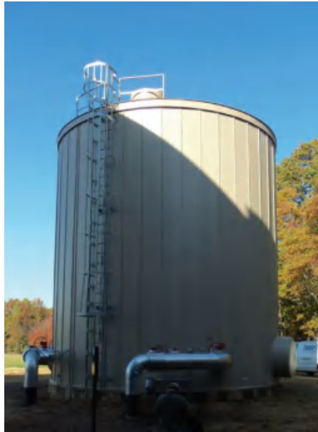
FIGURE 16.8 Chilled water storage tanks at Princeton University, Princeton, New Jersey.
