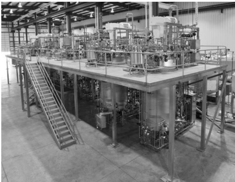
FIGURE 12.18 A 20,000 L insulin fermentation train under construction with mezzanine access. (Courtesy of ABEC, Bethlehem, PA.)
