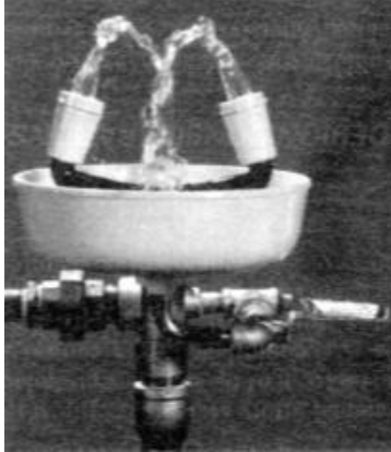
FIGURE 17.3 Stream from typical eyewash.
