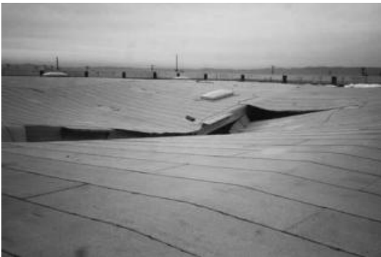
FIGURE 7.4 Heavy Snow Loads Allowed to Build on the Roof Can Lead to a Structural Collapse.
