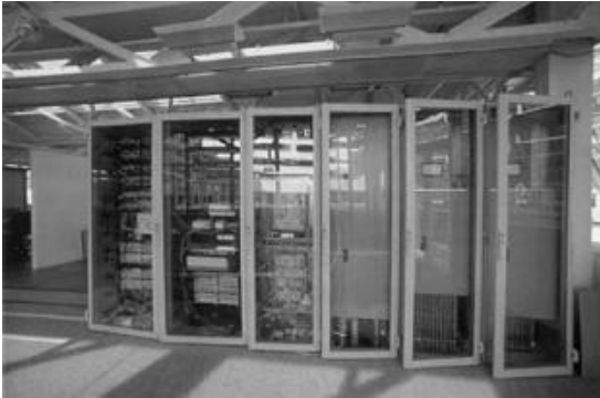
FIGURE 12.22 The Intelligent Workplace Demonstrates Distributed Satellite Closets Which Are Modular and Relocatable, Customized for Working Neighborhoods of 35–50 People, with Modular Racks Supporting Fiber, Data, and Voice Patch-Panels, Routers, Servers, Environmental Control and Security Modules. While Most 10,000 ft 2 Neighborhoods Might Need Two Modular Closets, This Laboratory Demonstrates Extensive Power Submetering and Competitive Control Systems Requiring Six Closets.
