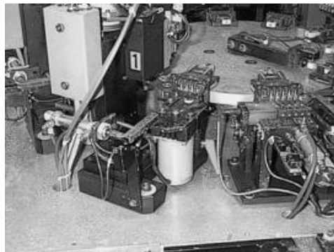
FIGURE 7.10 Corrosion of Equipment Occurs Rapidly after Exposure to Sea Water Carried Inland by a Hurricane.
