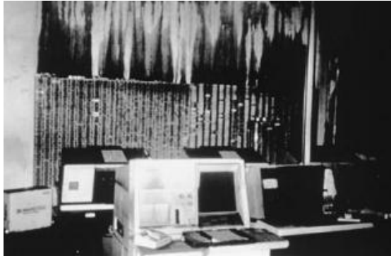
FIGURE 7.9 If Untreated, Electronics Exposed to Heavy Concentrations of Acidic Soot Will Be Ruined within Hours.
