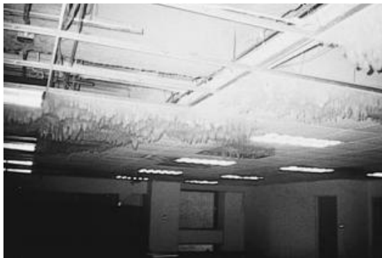
FIGURE 7.13 Fungus Growing on Water Saturated Ceiling Tile after Two Weeks Would Have Been Much Easier to Prevent Than to Clean.
