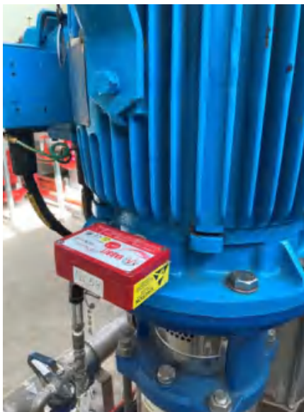
Figure 3.1 Internet-of-Things (IoT) sensor installed on pump set for condition monitoring.
