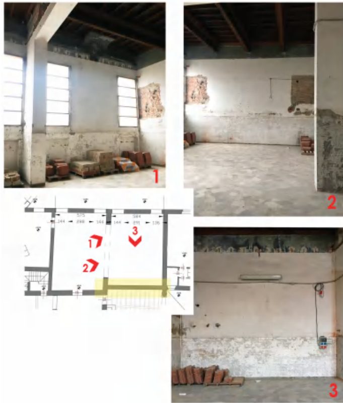
Figure 2. Internal views of the room. The picture 3 represents the wall selected for the tests.
