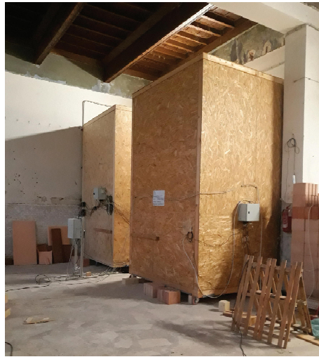
Figure 5. Internal view of the room, with the two boxes tied up to the studied wall.
