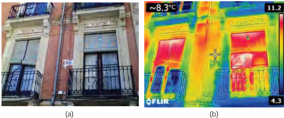
Figure 1. (a) Placement of the thermal flow plate and probes on the exterior face of the facade; (b) Thermographic image of the facade.
