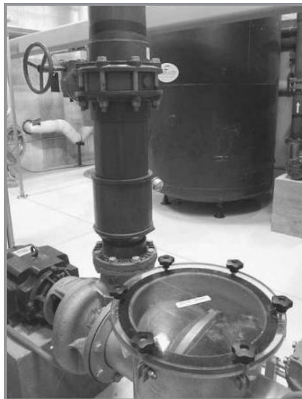
Figure 8.6 The filter room at an aquatic facility.
