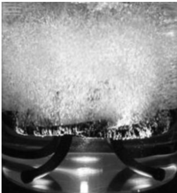
Figure 13.5 Fine bubble membrane diffusers in an aeration tank (Courtesy of Wikipedia; http://en.wikipedia.org/wiki/File:DualAir_Grid_System.jpg ).
