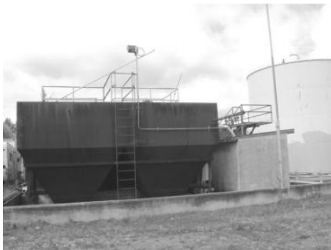
Figure 15.14 Upflow settling basins ( http://yosemite.epa.gov/R10/CLEANUP.NSF/9f3c21896330b4898825687b007a0f33/8572edc919ef3f31882569f50002f069/$FILE/P4140080.JPG ).
