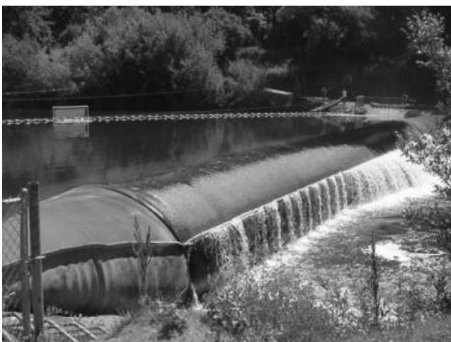
Figure 3.11 Inflatable rubber dam (Courtesy USGS).
