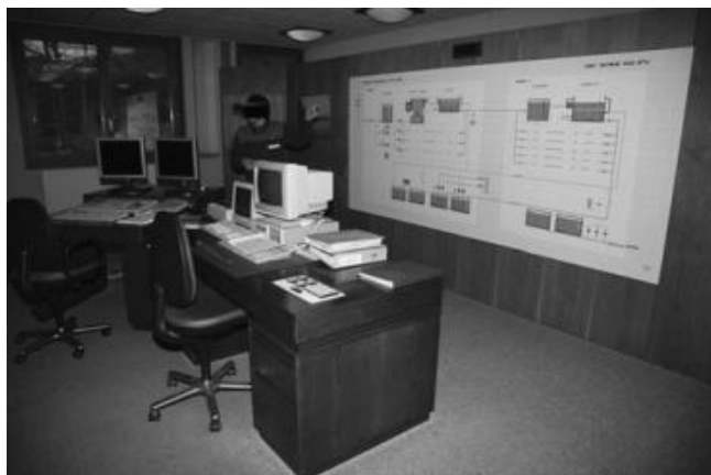
Figure 16.11 Control room and schematics of the water purification plant to Lac de Bret, Switzerland ( http://en.wikipedia.org/wiki/File:Usine_Bret_MG_1638.jpg ).
