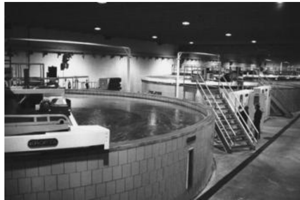
Figure 15.26 World's largest DAFF 37.5 MGD potable water treatment plant was built in 1986 in Pittsfield, MA (Wang, 1991).
