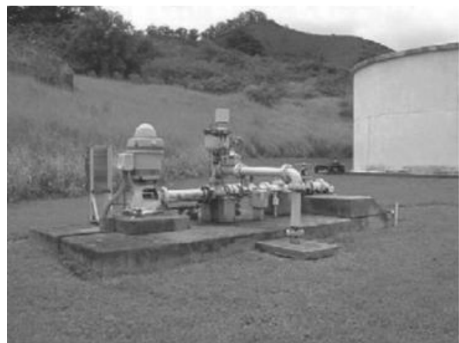
Figure 3.15 Well and 190,000 gal (719,150 L) Tank, Maui, HI (Courtesy of the Department of Water Supply, Maui County, HI).
