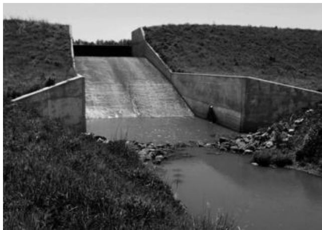
Figure 2.5 Concrete spillway in dam (Courtesy of the Department of Water Supply, Maui County, HI).
