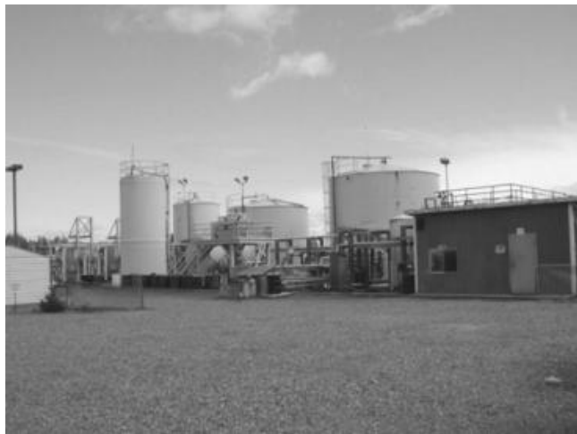
Figure 11.7 General view of a groundwater treatment plant, http://www.epa.gov/waterinfrastructure/pdfs/brochure_si_sustainin_gournationswaters.pdf .
