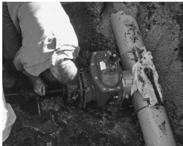
Figure 6.6 Cast-iron gate valve being installed on a new connection to a fire hydrant (Source: http://en.wikipedia.org/wiki/Image:MunicipalGateValve.JPG ).
