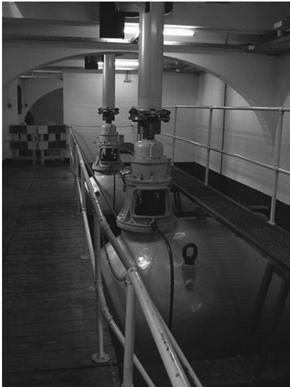
Figure 8.1 Pumping station Van Sasse in Grave, the Netherlands (Source: http://en.wikipedia.org/wiki/Image:Gemaal_van_sasse_interieur.jpg ).
