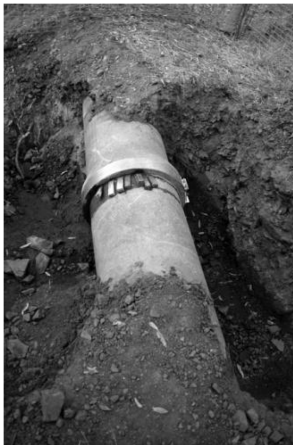
Figure 5.23 Concrete water pipe (Source: http://upload.wikimedia.org/wikipedia/commons/2/2e/Concrete_water_pipe.jpg ).
