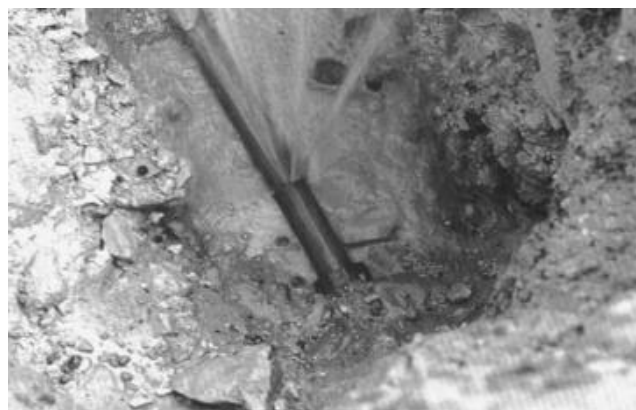
Figure 4.3 Water leakage from a crack in a water pipe.
