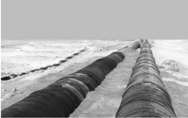
Figure 5.22 The dual 1,600-mm desalinated water transmission line in Abu Dhabi, UAE. The pipes are 250 km long. The pipes are ductile iron laid above ground level with bitumen/zinc coating (Source: http://www.water-technology.net/projects/shuweihat/shuweihat4.html ).
